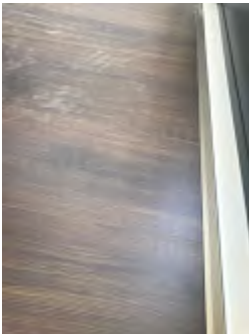
Ghosting in up stairs bedroom.JPG 2082K
