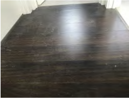
Ghosting near Main bathroom.jpg 1101K
