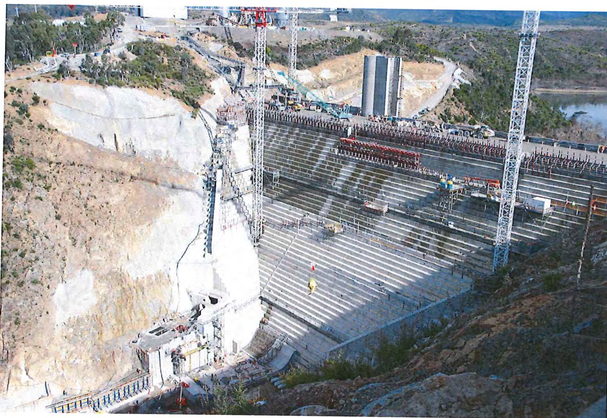
Photograph 3.3 The downstream face of the dam as at 15 August 2012. The RCC deck level was at RL 532, which is 20 m below the crest level of the primary spillway.
