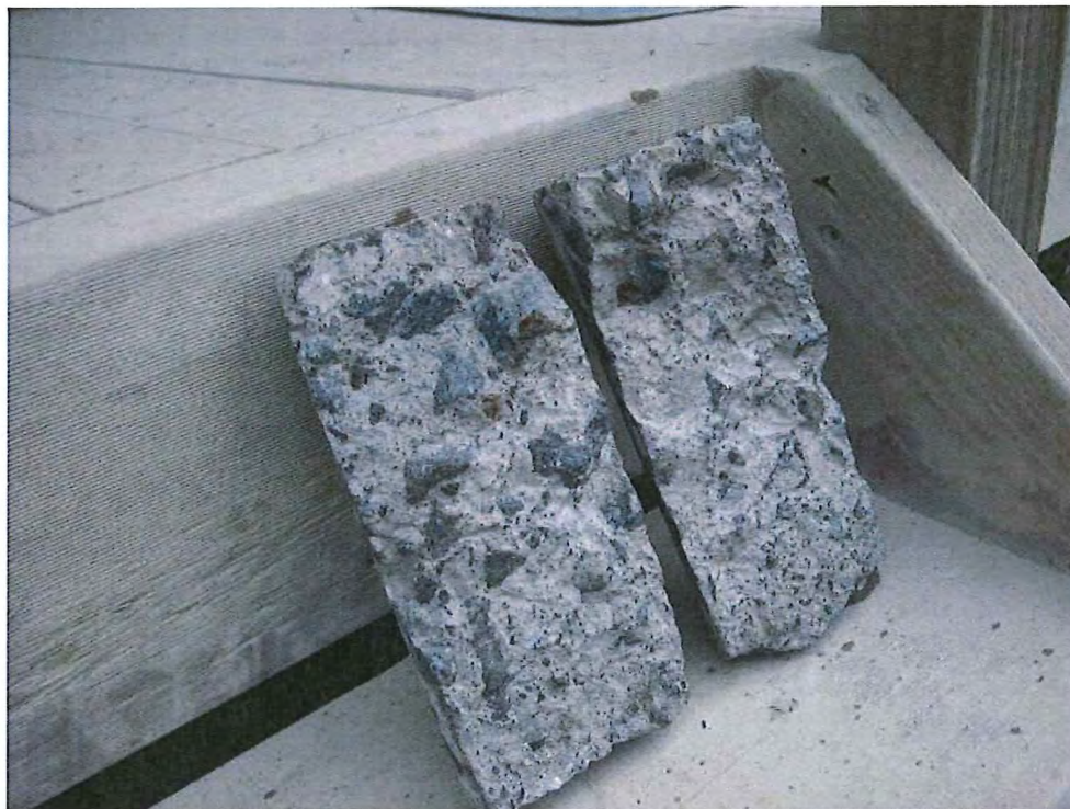
Photograph 5.3 Drilled core along the lower of the two horizontal cracks in the downstream face. The joint surface seems to be at the bottom of the cores – the top of the core is the vertical face of the step. The crack has initiated off the joint at the outer face (see Photograph 5.4).
