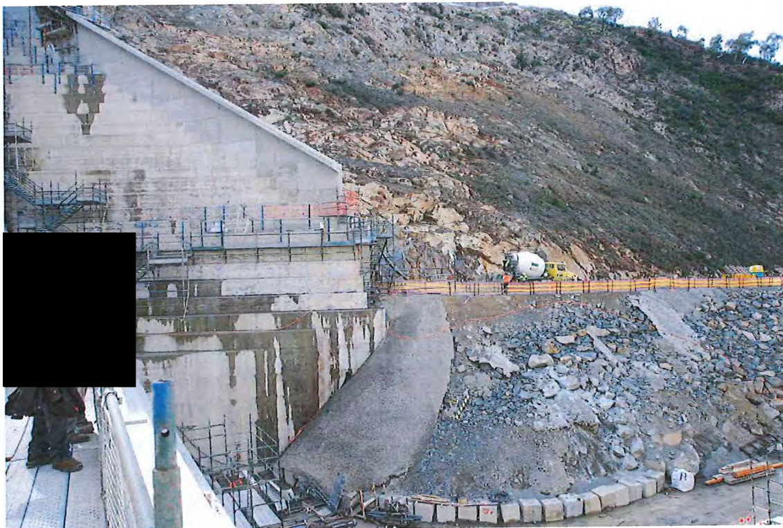
Photograph 3.2 The left hand side of the spillway's stilling basin, showing the way the outlet of the 3 m diameter conduit of the Stage 2 diversion works is now holding up progress on this side of the stilling basin.
