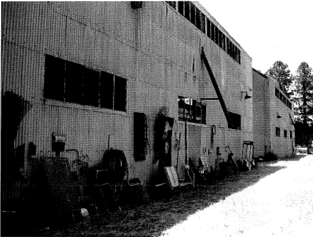
Figure 110 The rear (east) wall of Machine Bay II. The adjoining building (to the north) is Machine Bay III.
