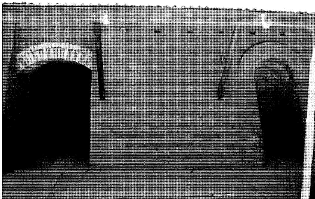
Figure 86 Kiln wickets – the opening at left has been altered to enable forklift access and the bricked-up the opening at right is as originally built.
