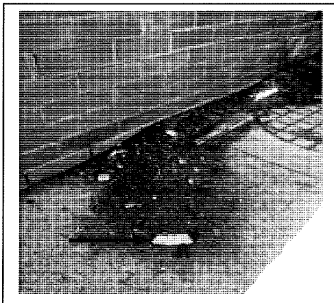
Photograph 13: Scattered sheeting debris** (in various locations) Refer Sample: 2810 - 40 - A14
