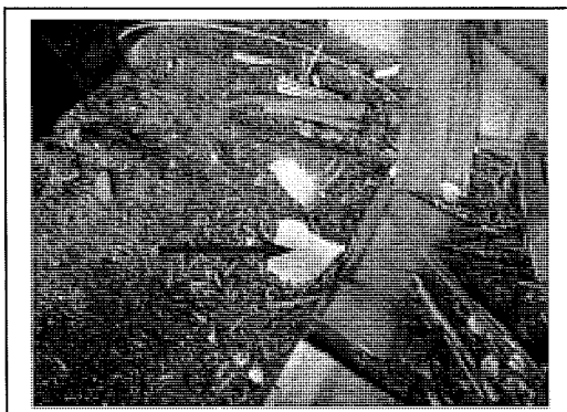
Photograph 15: Debris to small chimney at entrance Sheet Refer Sample: 3617 - 103 - A2
