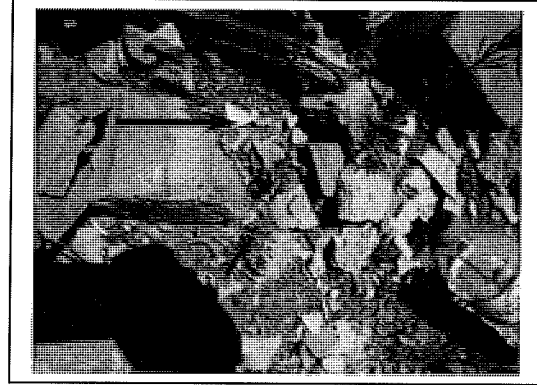
Photograph 18: Sheet debris to soil adjacent FH2 building Refer Sample: 3617 - 103 - A7
