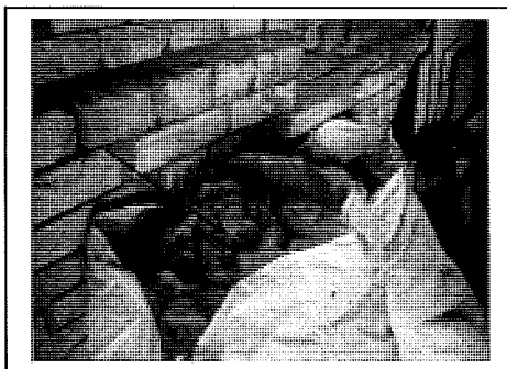
Photograph 23: Lose SMF in bags presumed to contain asbestos throughout kilns Refer Sample: 3617 – 103 – S1
