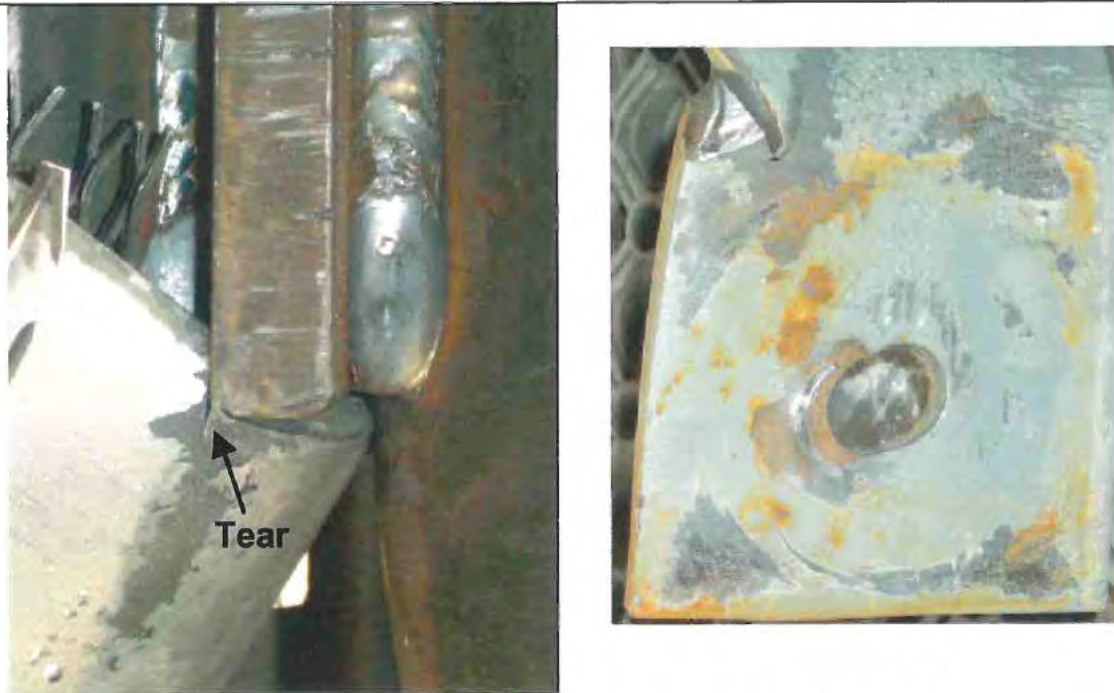
Figure 32 – Tearing of End Plates and Elongation of Bolt Holes
