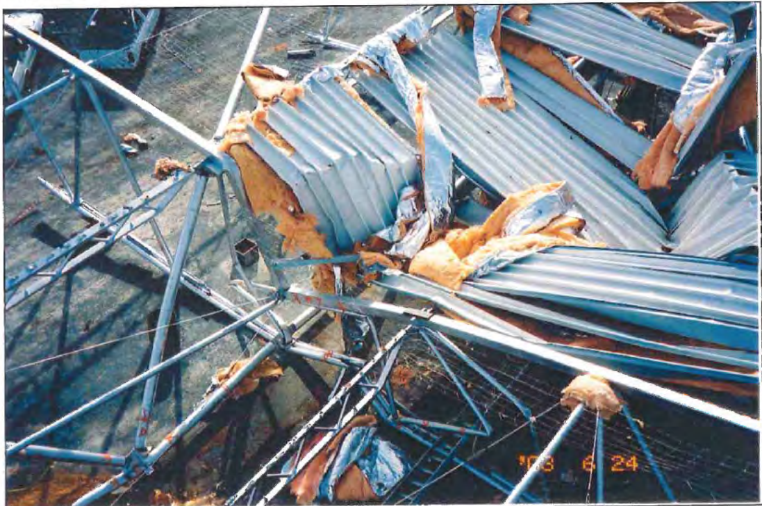
Figure A6: View from above, over central section of SF7. Note the buckled top chord.
