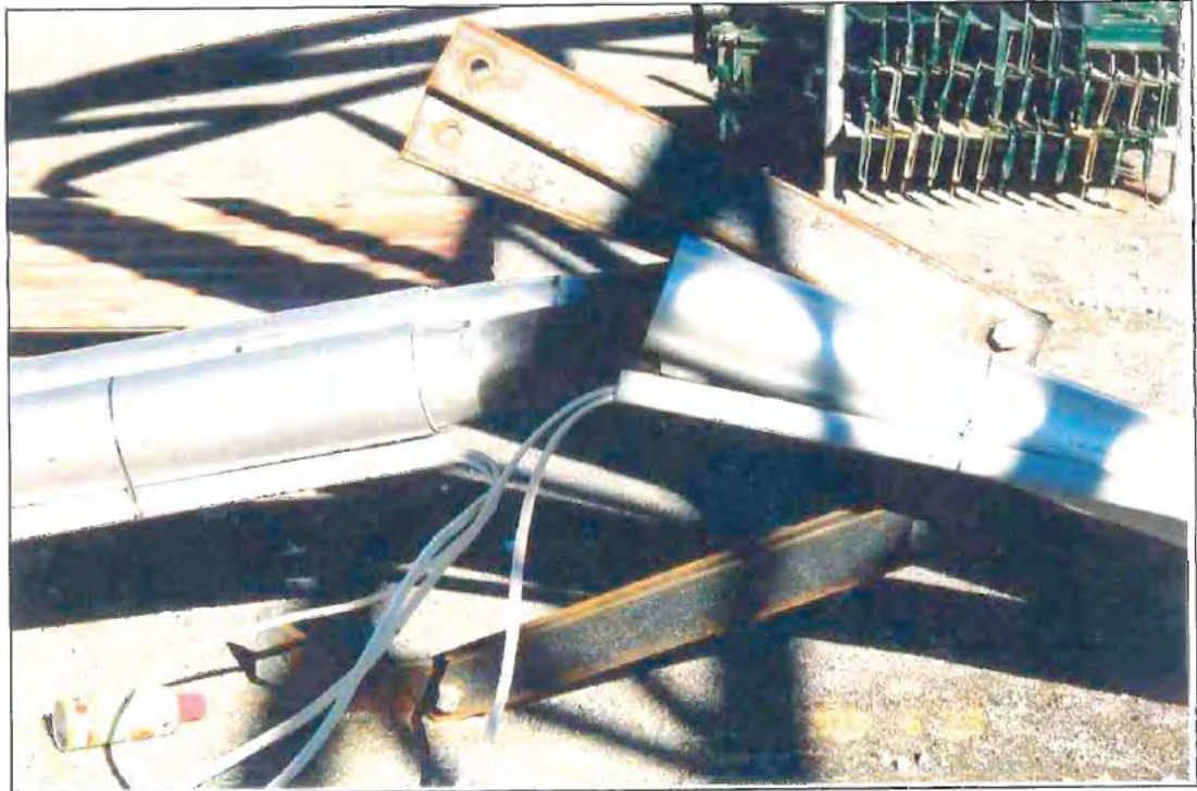
Figure A3: Failed gap lock plate on SF4.
