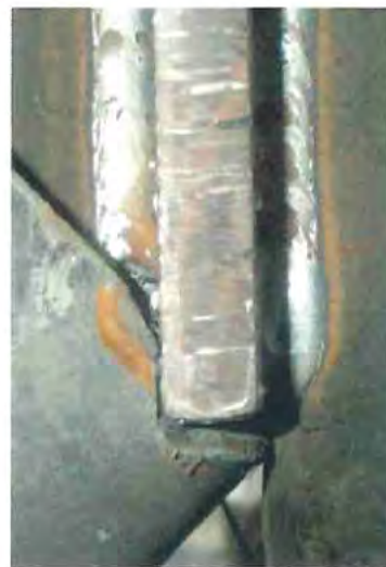
Tearing of end plate
