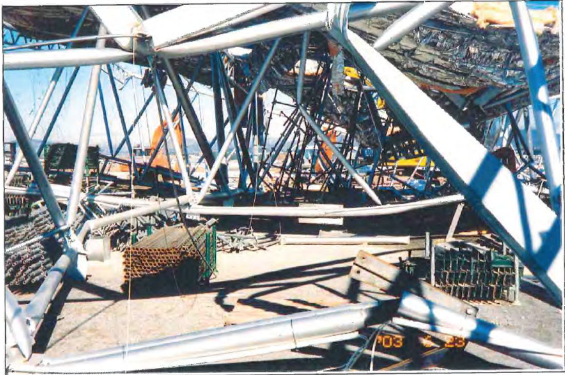
Figure A5: Failed gap lock plate on SF5.
