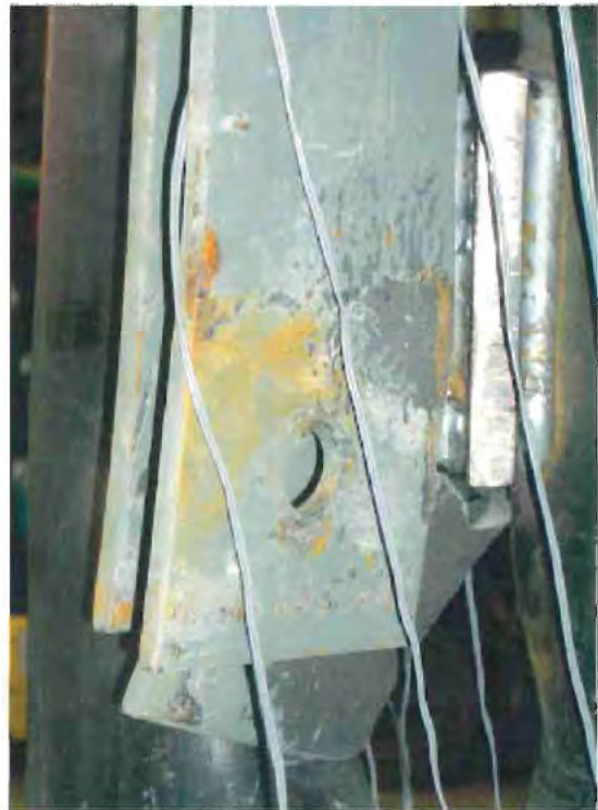
End plate at failure
