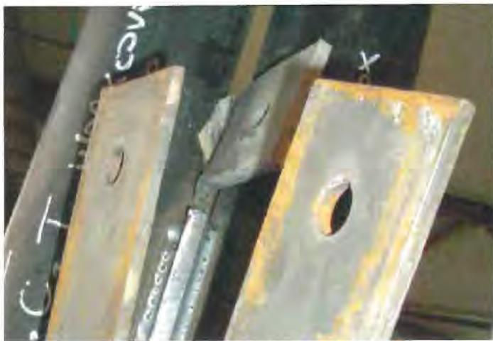
(a) Failed bolt Missing
