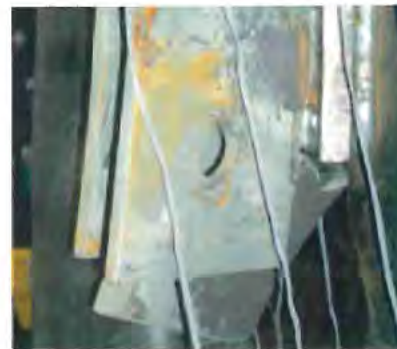
(b) Missing Bolt
