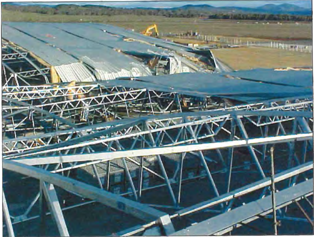
Figure A1: Global View of the failed structure. Note 3.5 bays have had roof sheeting applied.
