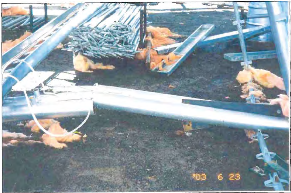
Figure A2: Failed gap lock at SF6
