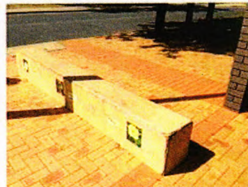
Seating walls badly damaged - remove and replace where appropriate with more durable product
