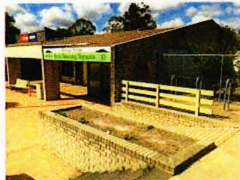
Non compliant ramp + stair limit access into shopping centre from adjacent bus stop - replace with new by recapturing fenced space beside building
