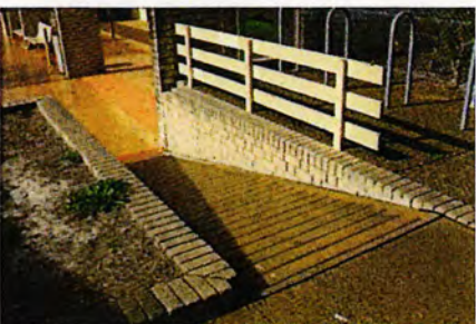
Non compliant and unsafe ramp adjacent to steps
