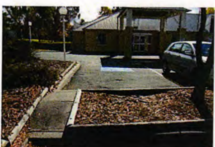
Removal of the kerb on both sides of the dividing planter bed and replacement with a accessible path would provide desire line access to and from the aged care facility
