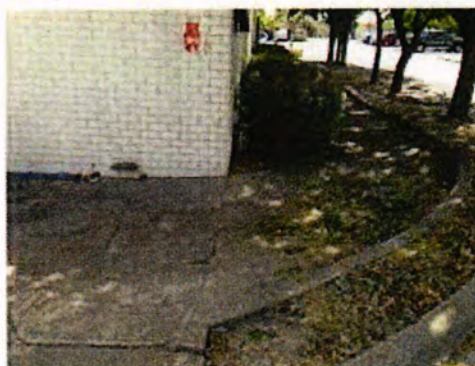
Cracked and uneven paving + drainage issues - install new at higher level to allow for adequate drainage to adjacent sump
