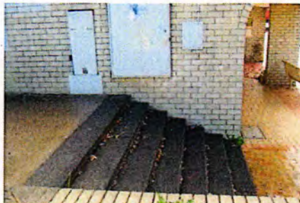
Alternative route via steps from a gap between the shops: steps are not compliant but could be rectified
