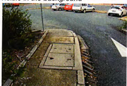
Current footpath access from the aged care facility: nil pram crossing
