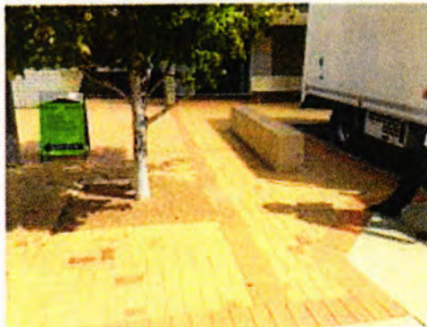
Brick paving in good condition - maintain and match / contrast with new paver if original no longer available
