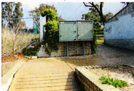
Power cubicles and fence to adjacent block that might preclude introduction of a compliant ramp in this location
