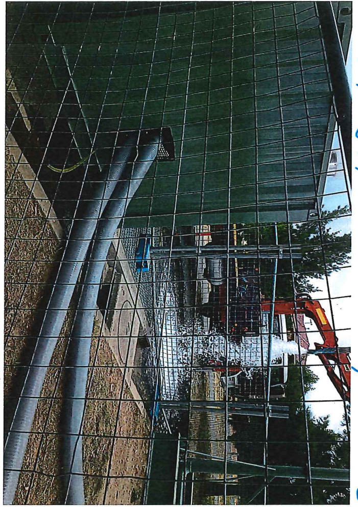
Pumps and pipes - Yonah's Pond W01392
