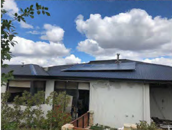
Scene of fire showing location of Solar Panels
