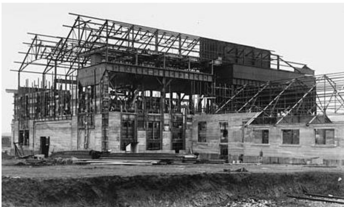
Figure 11 The Power House under construction, c. 1913-14: viewed from the south-west. Note rail line at right. Source: National Library of Australia.
