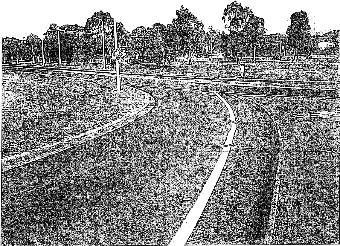
Figure 5 Pavement deterioration on westbound left slip
