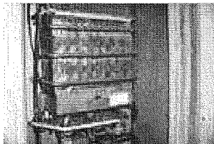
Asbestos panelling inside heater cupboard
