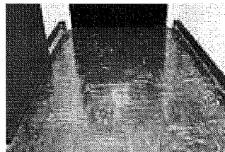
Asbestos containing floor tiles
