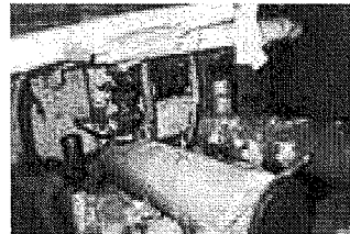
Damaged asbestos pipe lagging
