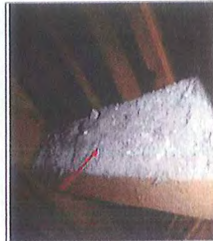
Photograph 6: Internal timber stud adjacent bathroom
