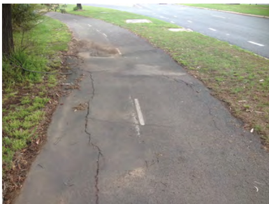
Poorly maintained shared path, Belconnen Way
