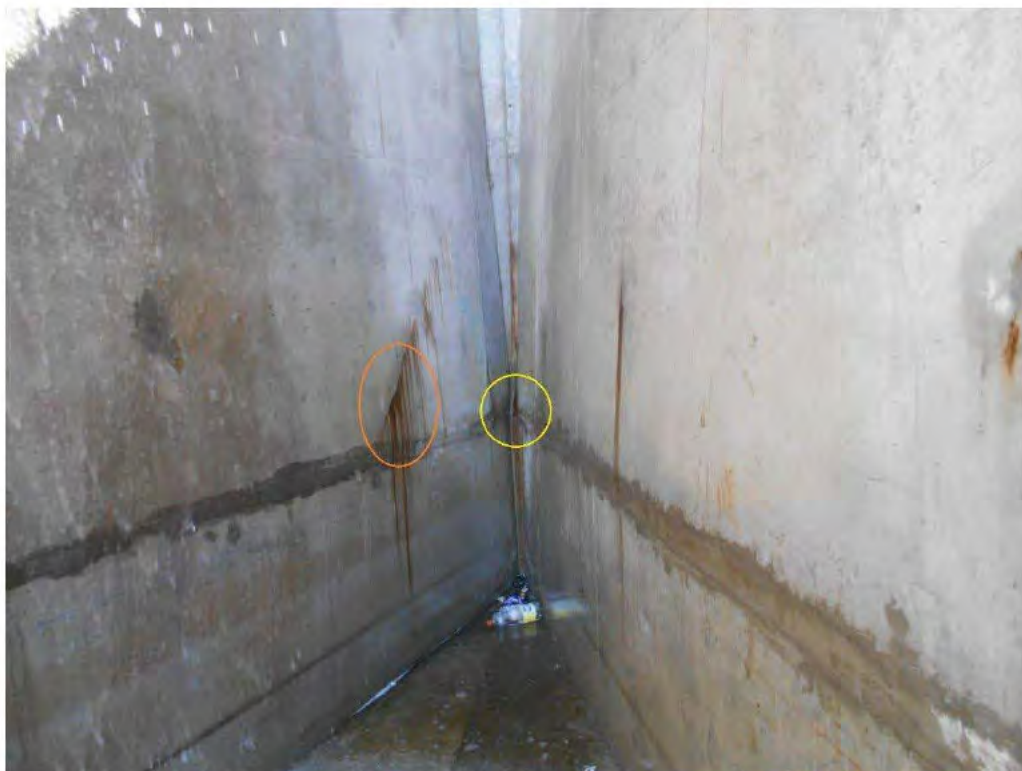
Photograph 17 – General view at the corner of LHS and RHS walls of the Bay 5. Close-up views of defects circled in orange and yellow are shown in Photograph 17 and Photograph 18.
