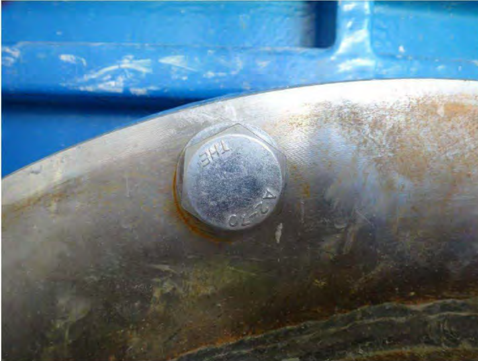
Photograph 37 - Close-up view of gate valve flange showing stained surface from carbon steel contamination.
