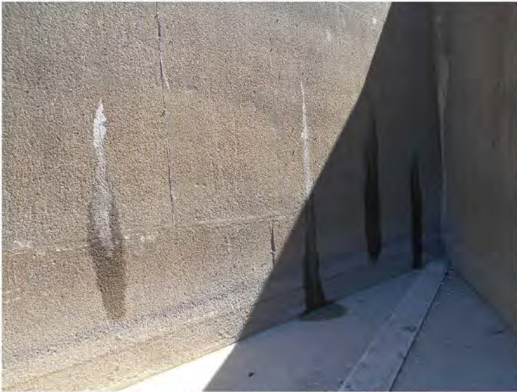
Photograph 23 – General view at the corner of LHS and RHS walls of the Bay 3. Note defects where minor seepage was evident.
