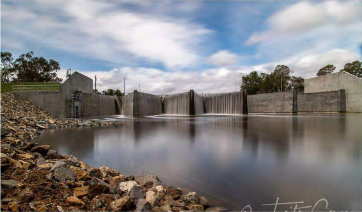
Photograph 43 (19 December 2019) – Downstream view of the weir. Spilling was not observed in Bays 1 (LHS end) and 2.
