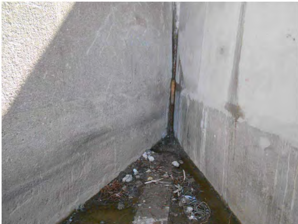
Photograph 25 – General view at the corner of LHS and RHS walls of the Bay 2. Note defects where seepage was evident.
