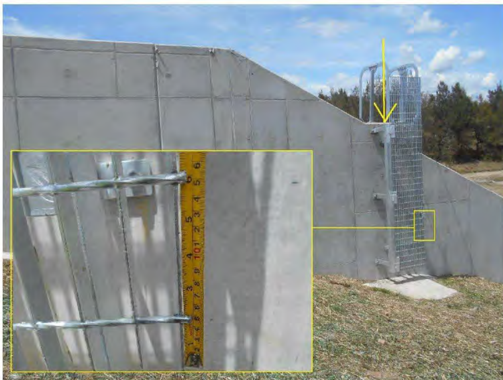
Photograph 14 – View of the ladder installed on the external face of the RHS abutment wall of the weir. There are several sharp edges (See inset). The bracket for installation of the “Recovery System” is shown in yellow arrow.
