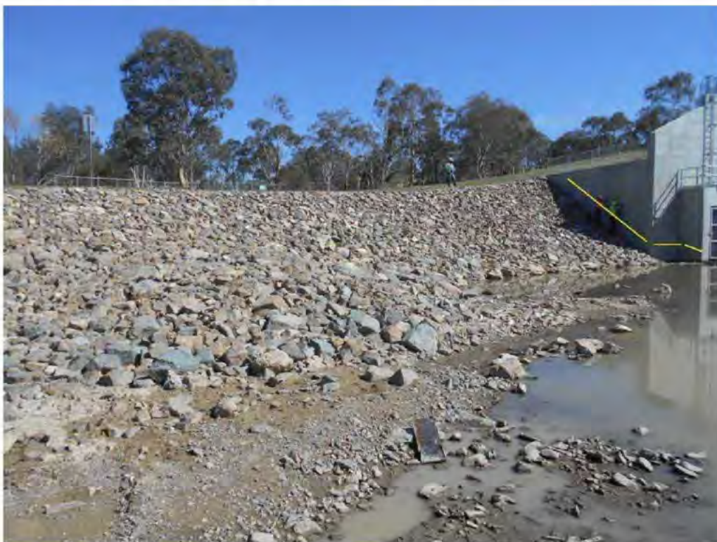
Photograph 10 – View of the RHS batter immediately downstream of the weir. There is no safe access to the downstream apron area from right abutment. Therefore, consideration should be given to providing a hand rail as shown in yellow, or similar acceptable arrangement.
