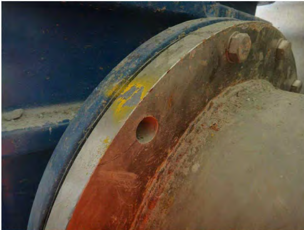
Photograph 39 – View of the upstream flange of the gate valve where one bolt was missing.
