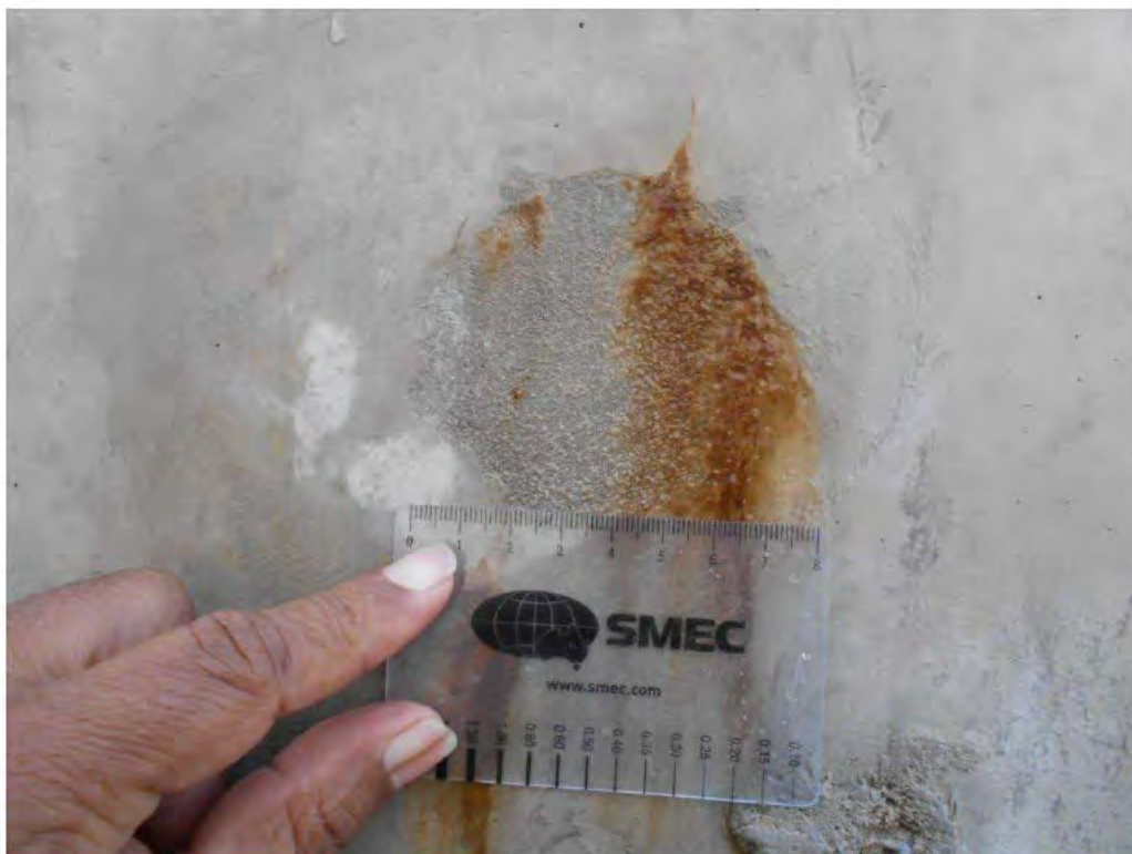
Photograph 21 – A close-up view of another defect in Bay 5.
