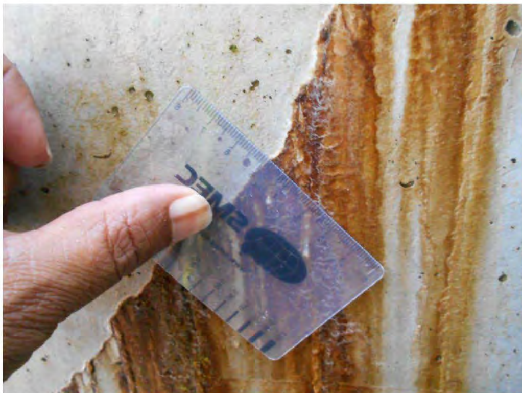
Photograph 18 – A close-up view of a defect on the RHS wall of the Bay 5 (Circled in orange in Photograph 17).
