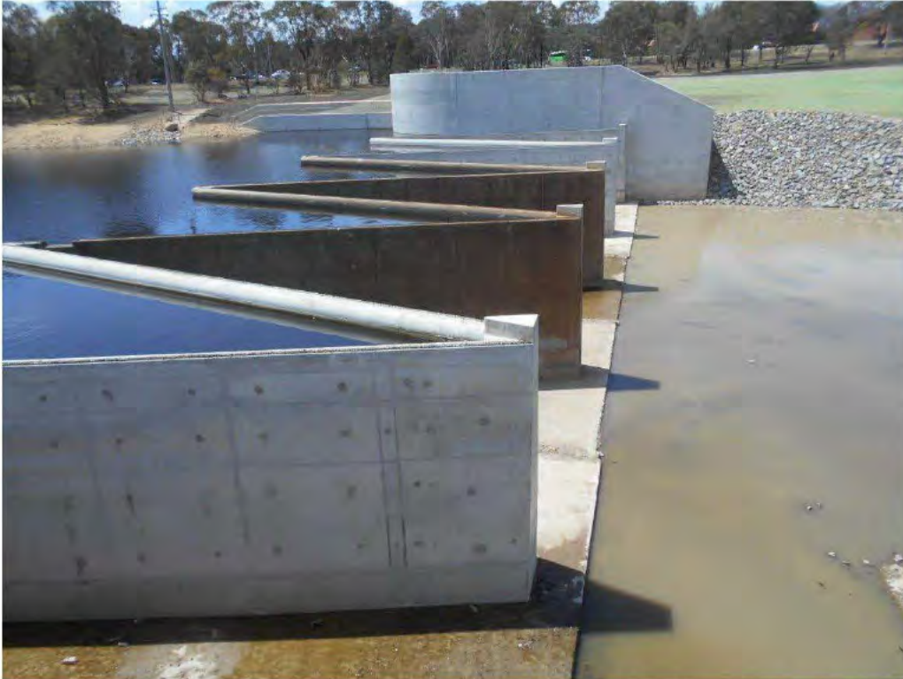
Photograph 3 – General view of the weir (Note: the water level of the downstream pool was lowered to facilitate the inspection).
