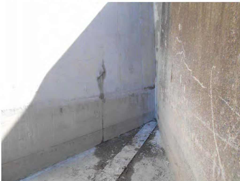
Photograph 22 – General view at the corner of LHS and RHS walls of the Bay 4. Note defects where minor seepage was evident.
