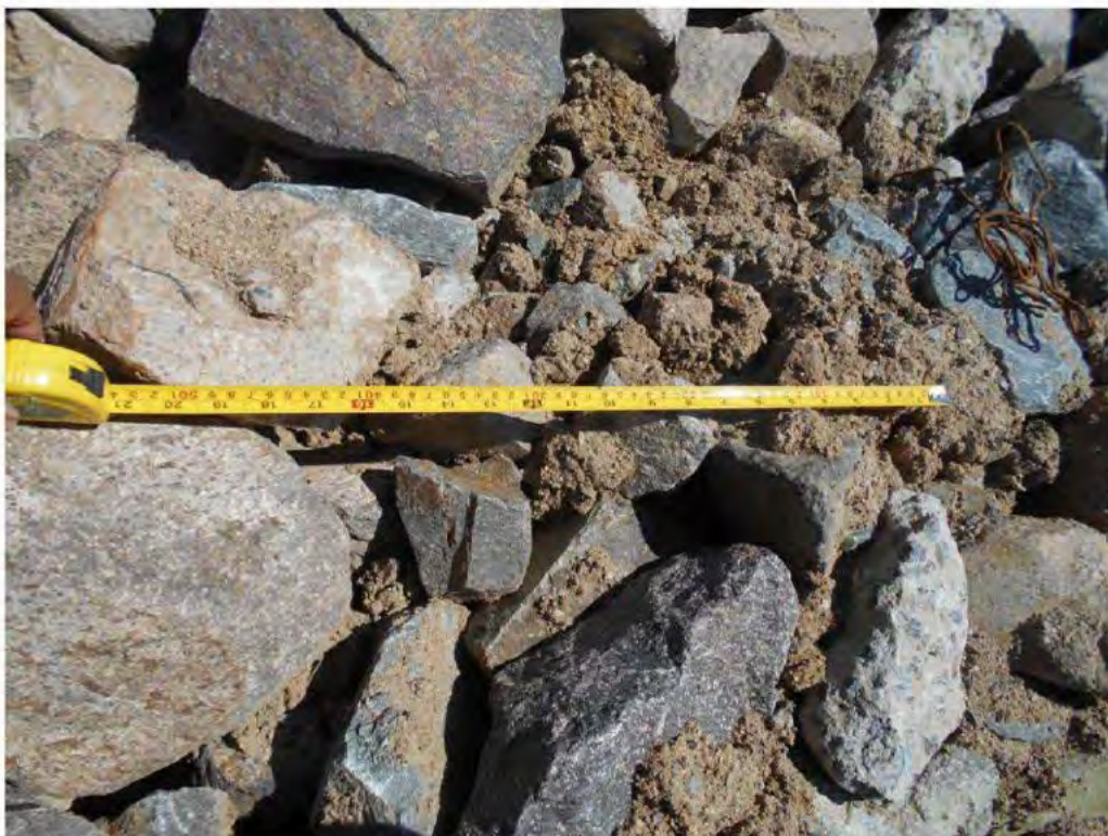
Photograph 11 – A close-up view of the tip-rap protection of the RHS batter referred to in Photograph 10. Note sand-like materials within the rip-rap protection which could be washed away during flood discharge.
