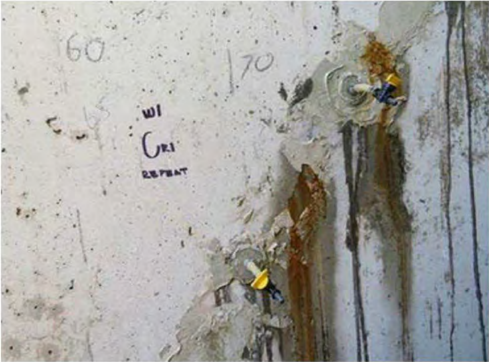
2. Water seeping through construction joint near contraction joint 5
