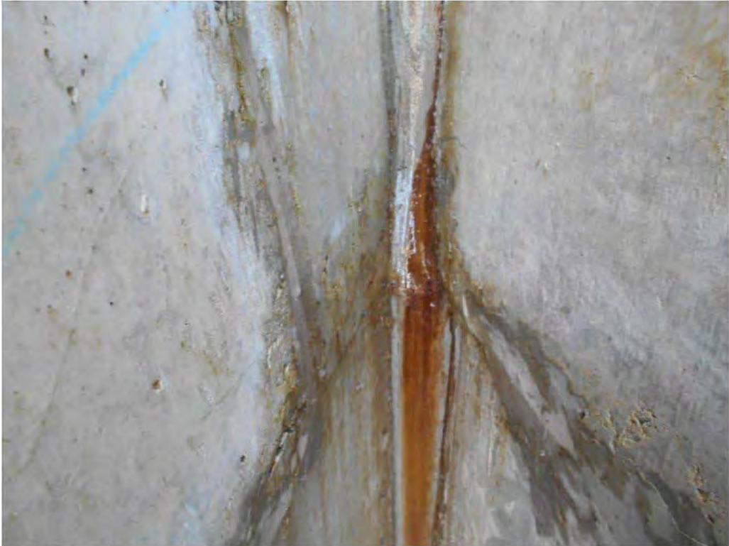
Photograph 19 – A close-up view of a defect on the RHS wall of the Bay 5 (Circled in yellow in Photograph 17).
