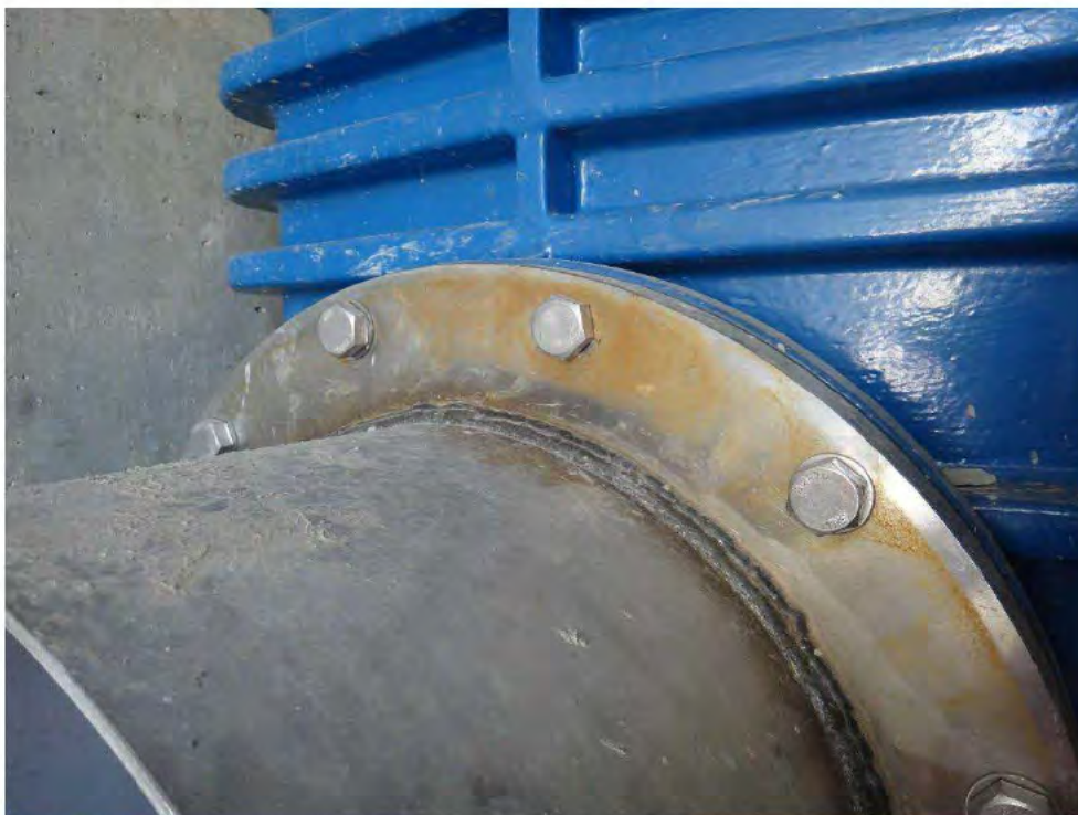
Photograph 40 – A Close-up view of the flange of the gate valve where there is evidence of stains from carbon steel contamination.
