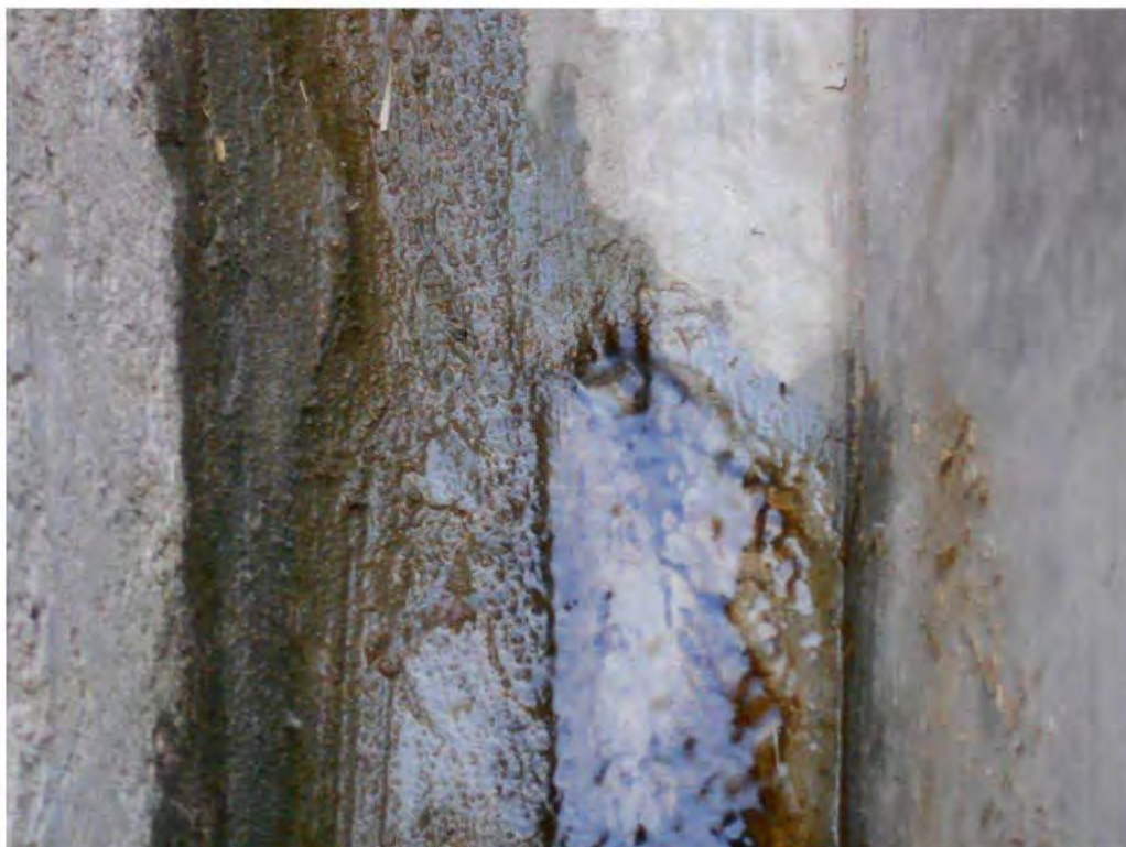
Photograph 26 – A close-up view of the defect at the corner of LHS and RHS walls of the Bay 2 and referred to in Photograph 25.
