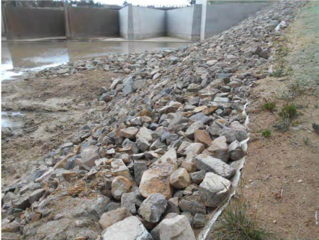
Photograph 33 – General view of the rip-rap protection of the LHS batter immediately downstream of the weir.
