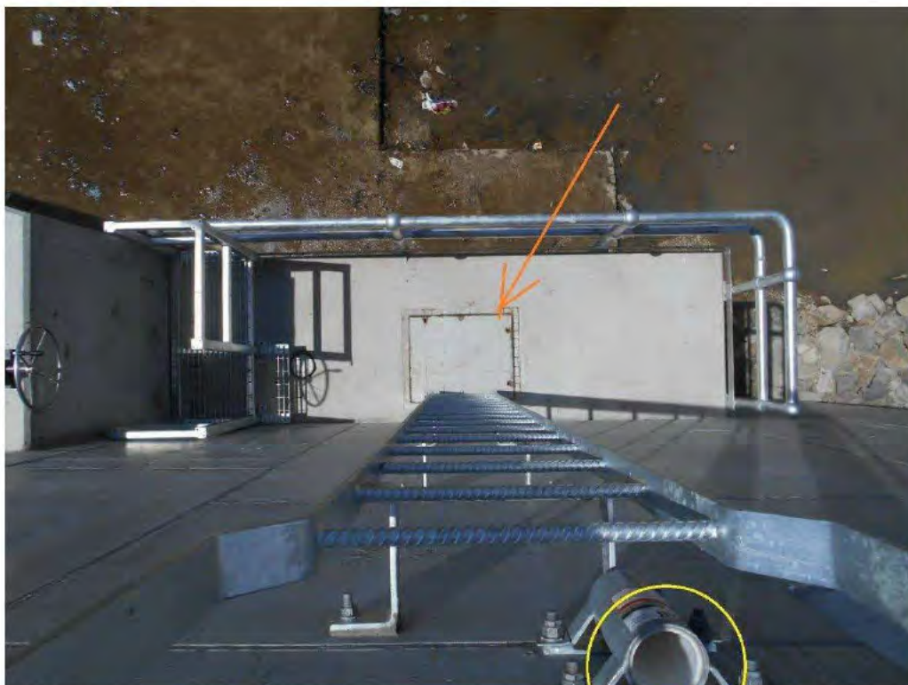
Photograph 15 – The ladder installed on the internal face of the RHS abutment wall of the weir, looking down from the top of the retaining wall.
