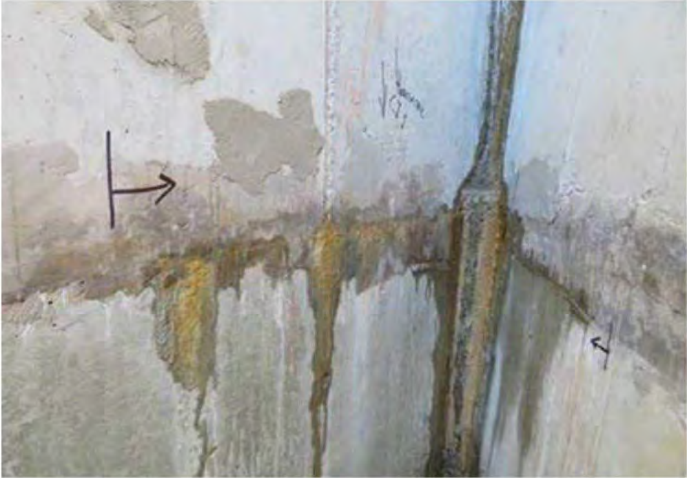
3. Water seeping through cracks on foundation slab (this is mainly on wall 9 and 10). Photograph is referring to wall 10, cracks 7 and 8 only.
