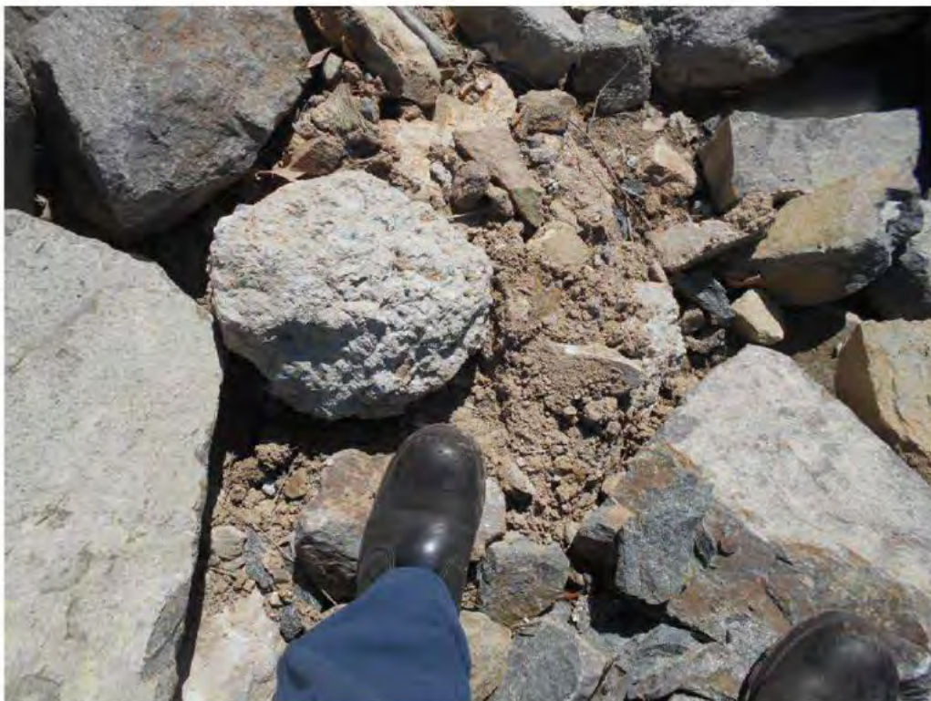
Photograph 12 – Another close-up view of the tip-rap protection of the RHS batter referred to in Photograph 10. Note sand-like materials within the rip-rap protection which could be washed away during flood discharge.
