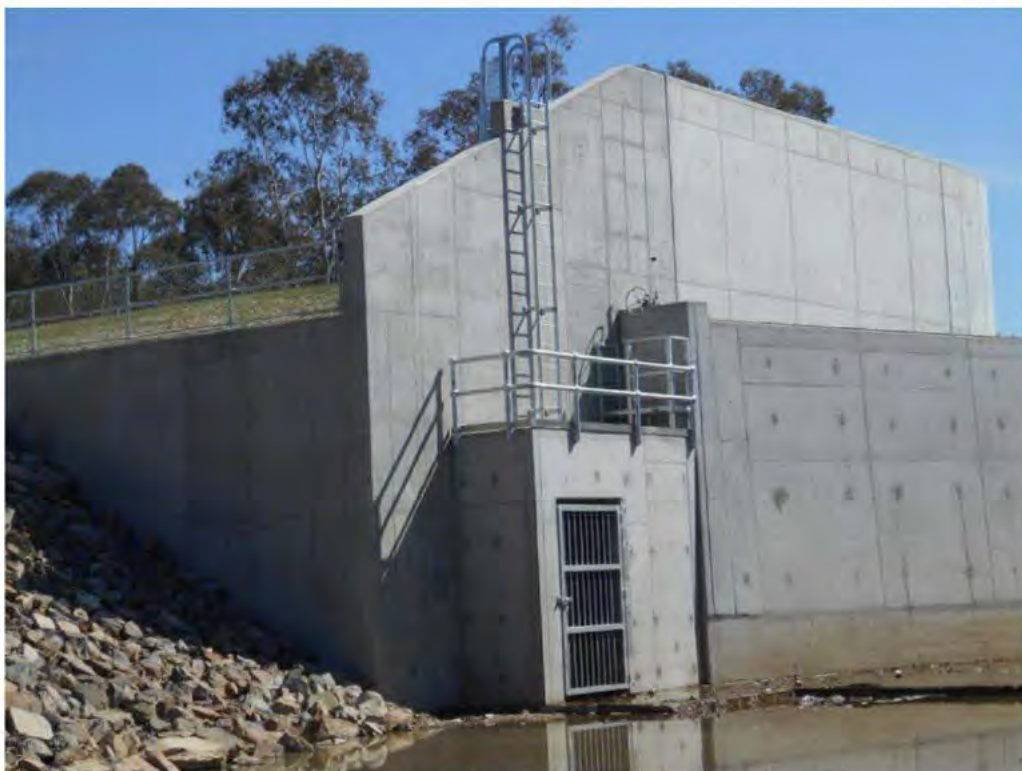
Photograph 13 – General view of the outlet valve chamber, valve operating platforms and access ladders. Note the ladder and bracket for the Devitt arm of the recovery system.
