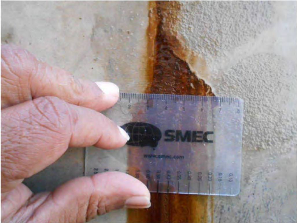
Photograph 20 – A close-up view of another defect in Bay 5.
