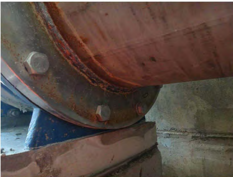
Photograph 38 – View of the underside of the stainless-steel pipework and flange showing improper preparation of works on stainless steel. There was evidence of surface corrosion. The bolt seen LHS of the photograph was found to be in loose state.
