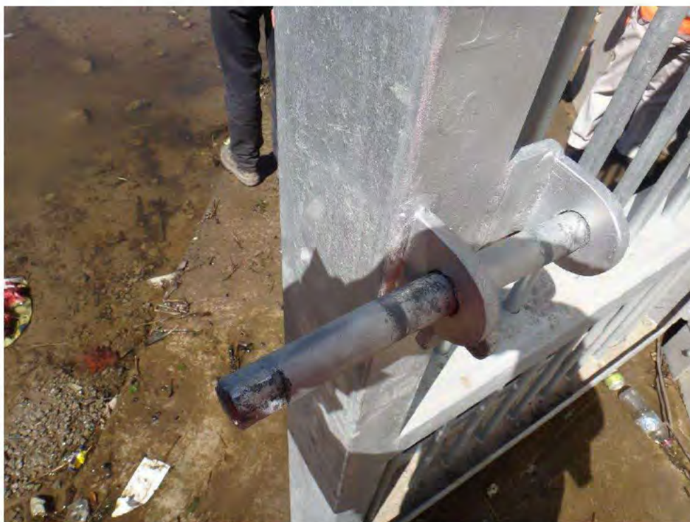
Photograph 36 – View of the locking bolt of the outlet valve chamber with evidence of wear and rubbing due to improper installation.
