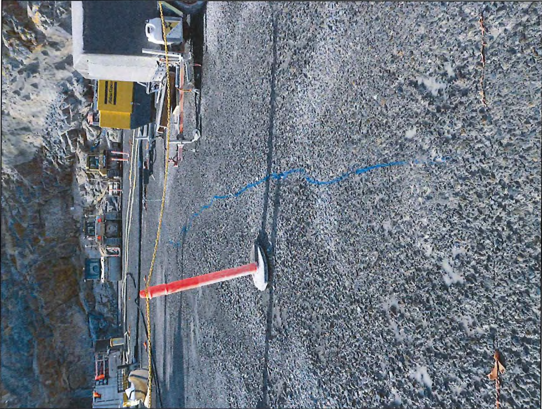
Photo A.6 – Cracking in Monolith F, looking towards left abutment (cracking outlined with blue paint).
