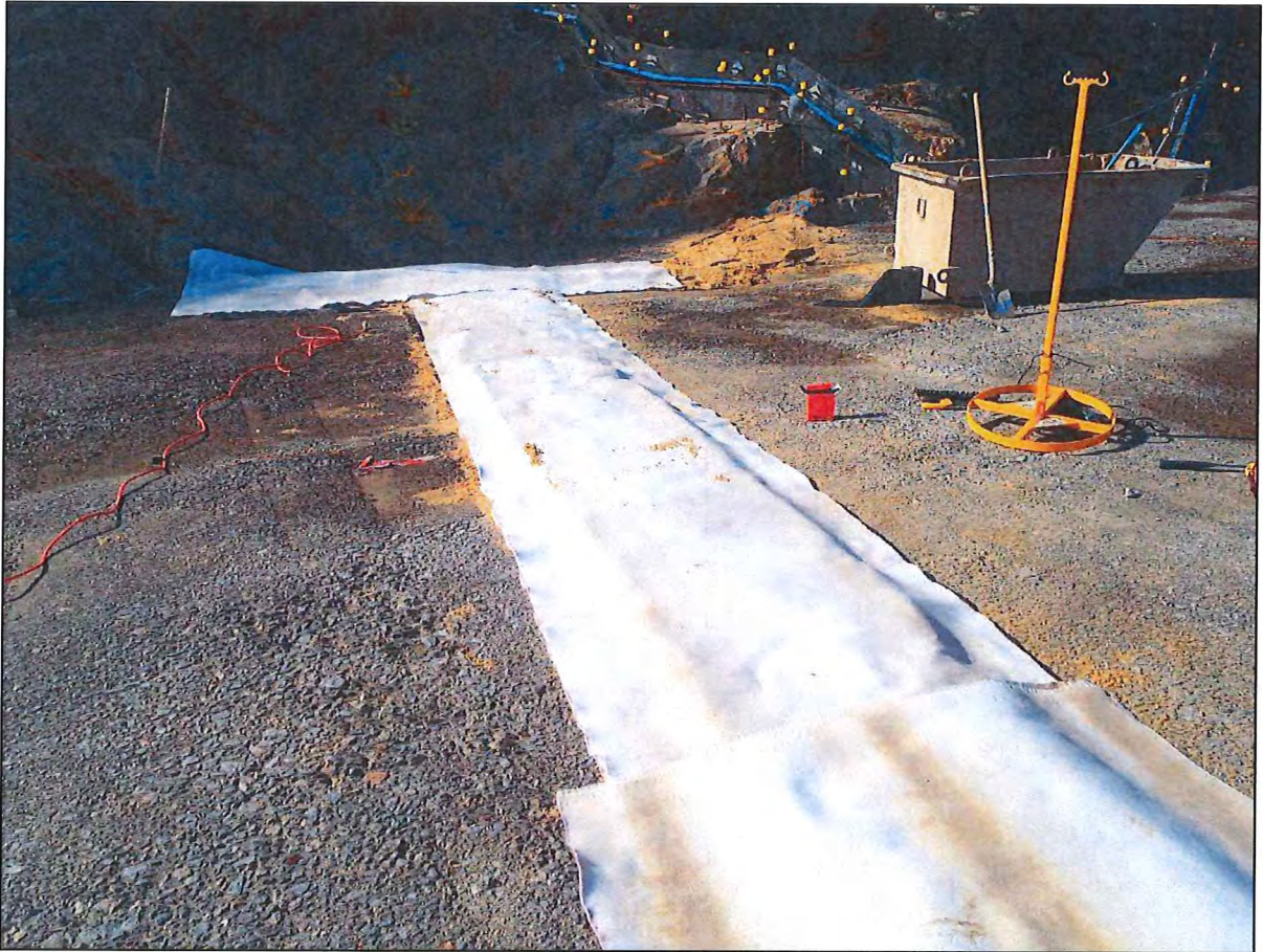
Photo D.1 – Sand crack stopper and strip drain being installed in Monolith D.
