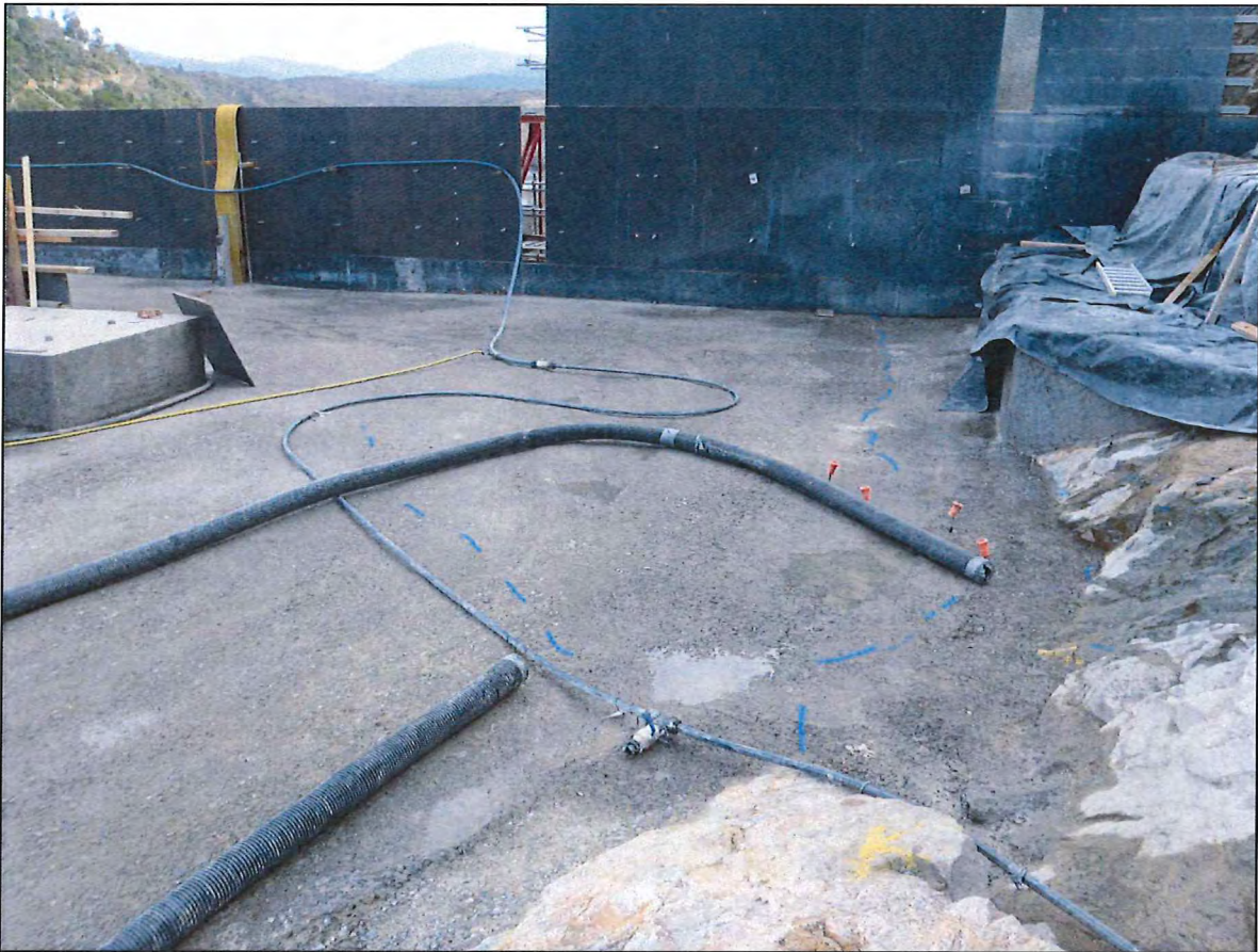
Photo A.4 – Cracking on upstream left abutment (cracking outlined with blue paint).
