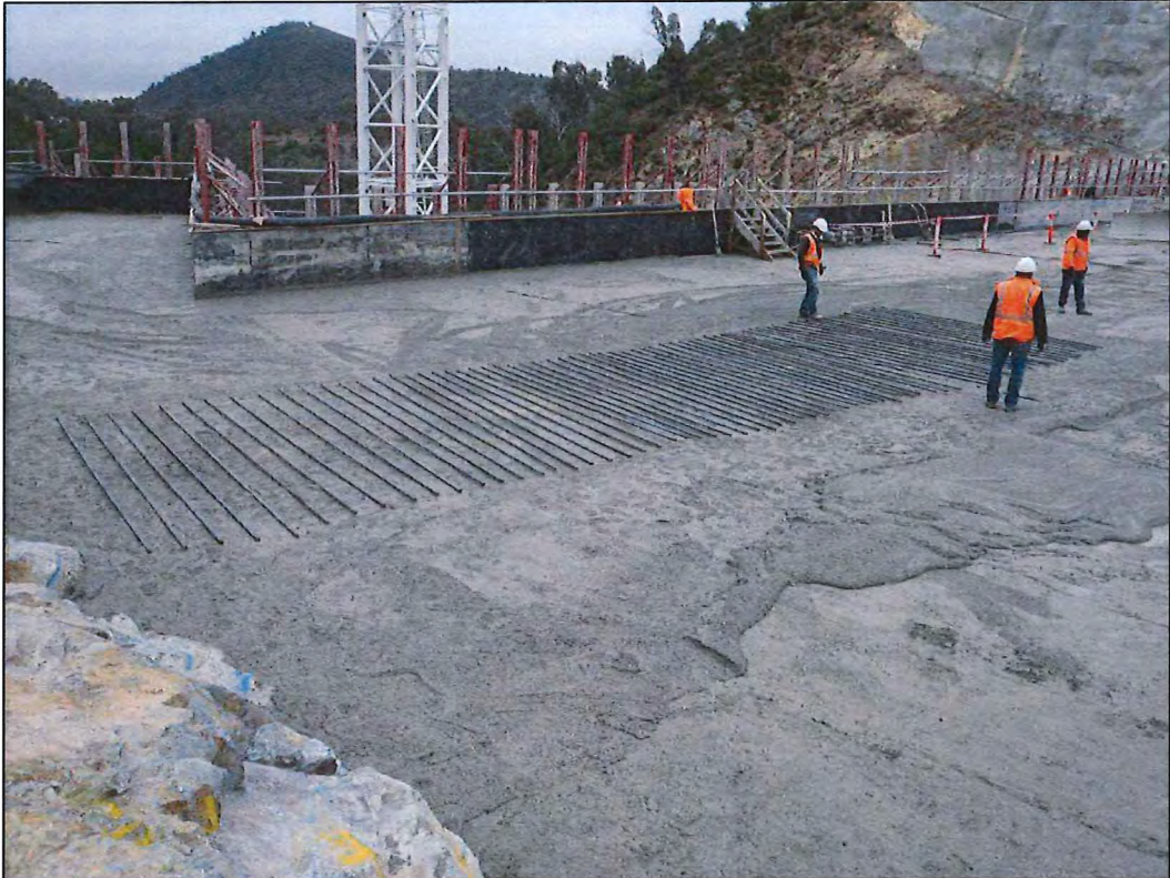
Photo D.6 – N28 reinforcement bars being installed on top of the cross valley cracks in Monolith D.
