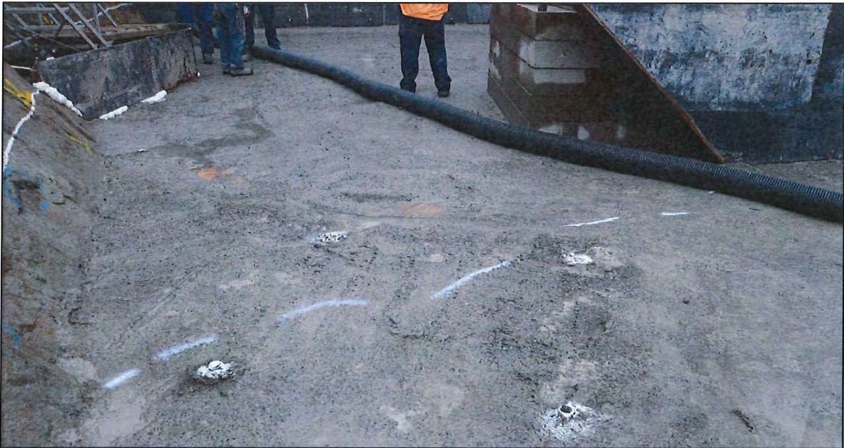
Photo A.5 – Cracking from right abutment to gallery blackout on RL510.9 (cracking outlined with white paint).
