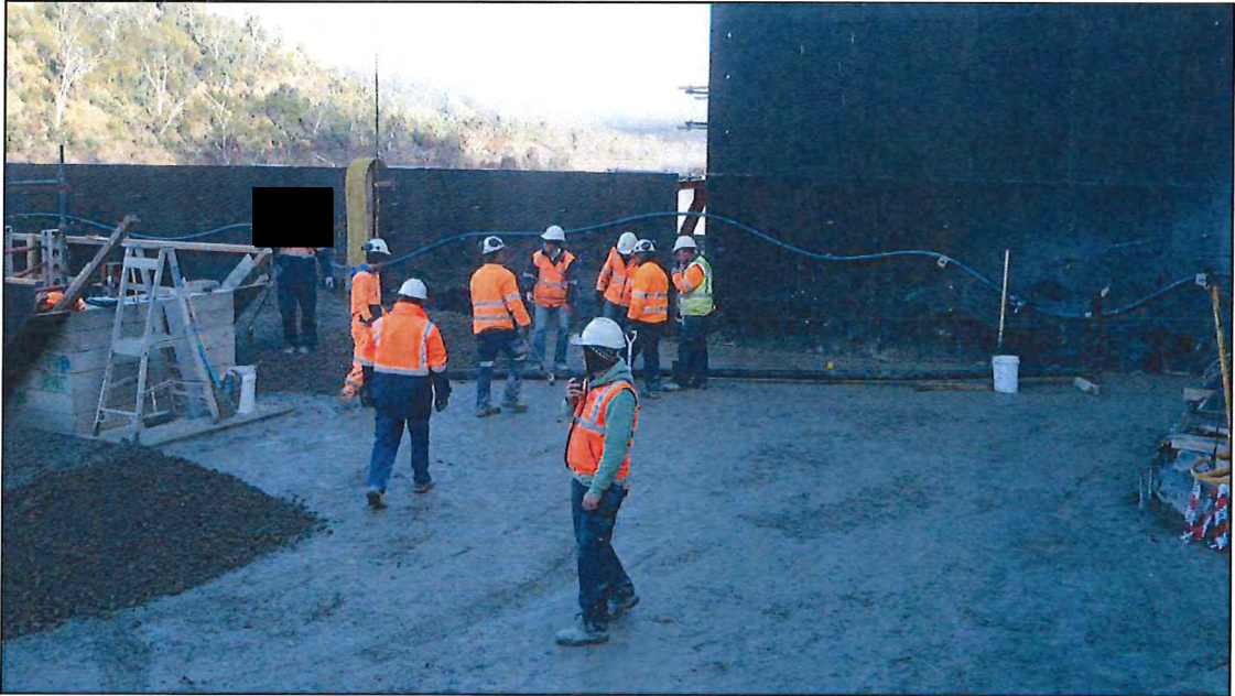
Photo D.9 – Installation of 100mm diameter riser pipe and drain connecting to gallery.
