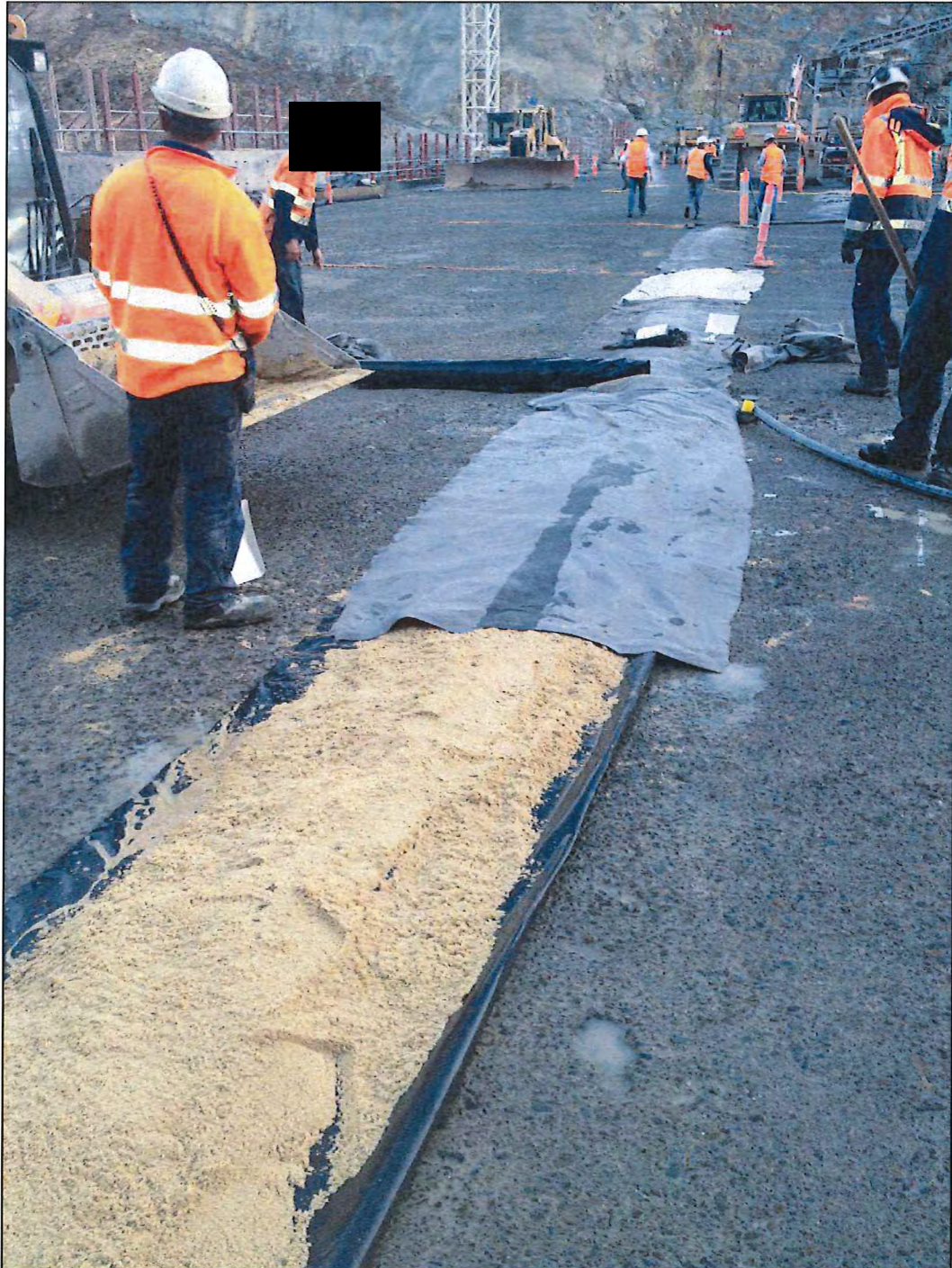
Photo D.2 – Sand crack stopper and strip drain being installed in Monolith E.
