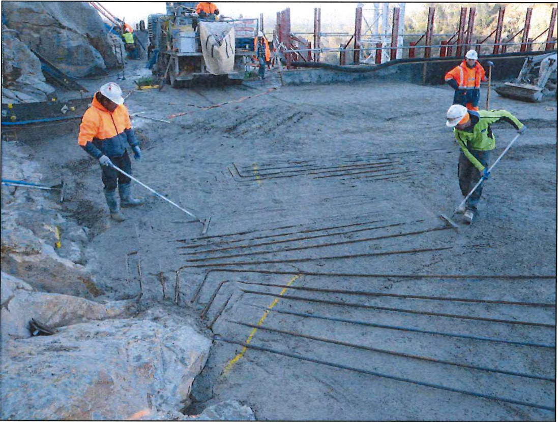
Photo D.8 – N24 cogged reinforcement bars installed across transverse crack on left hand abutment groin.
