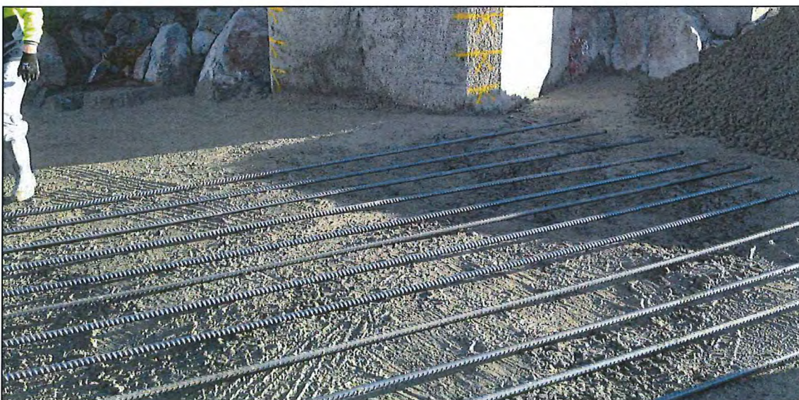
Photo D.11 – N28 reinforcement placed abutment to abutment on cross valley cracks, shown here in Monolith M.
