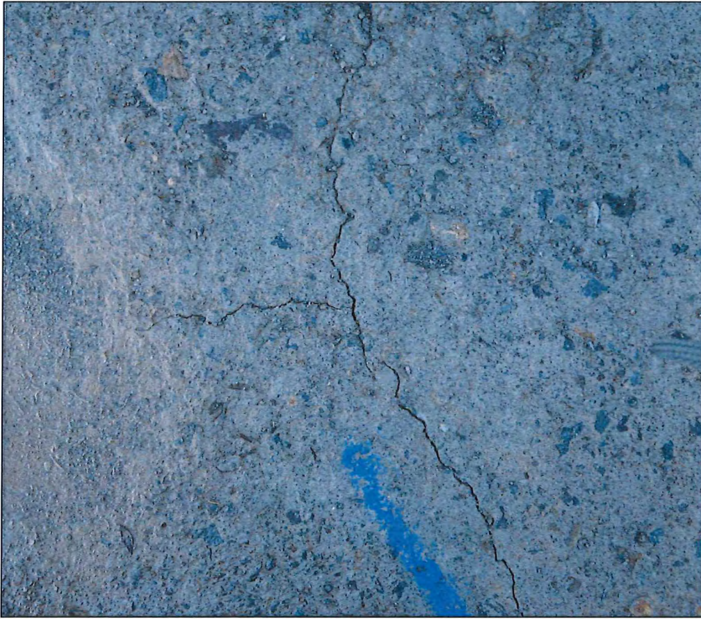
Photo A.2 – Bifurcation of upstream downstream crack with cross valley crack.
