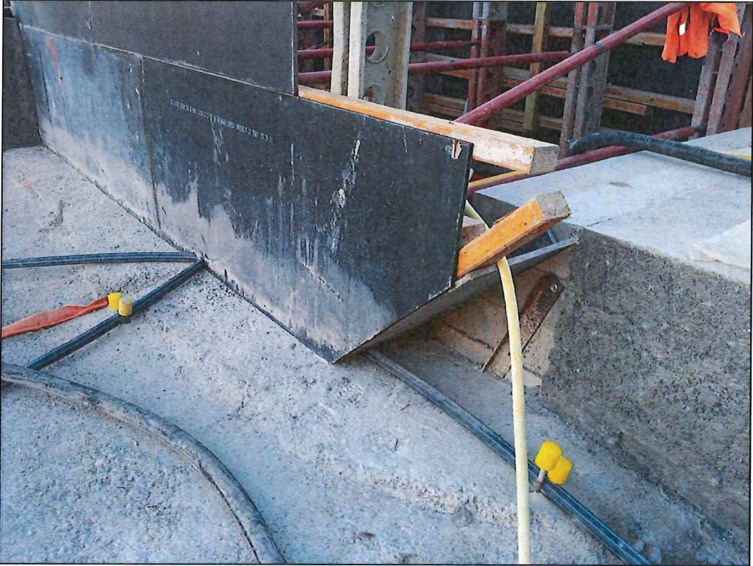
Photo D.4 – Drain pipes connecting strip drains to left hand gallery.
