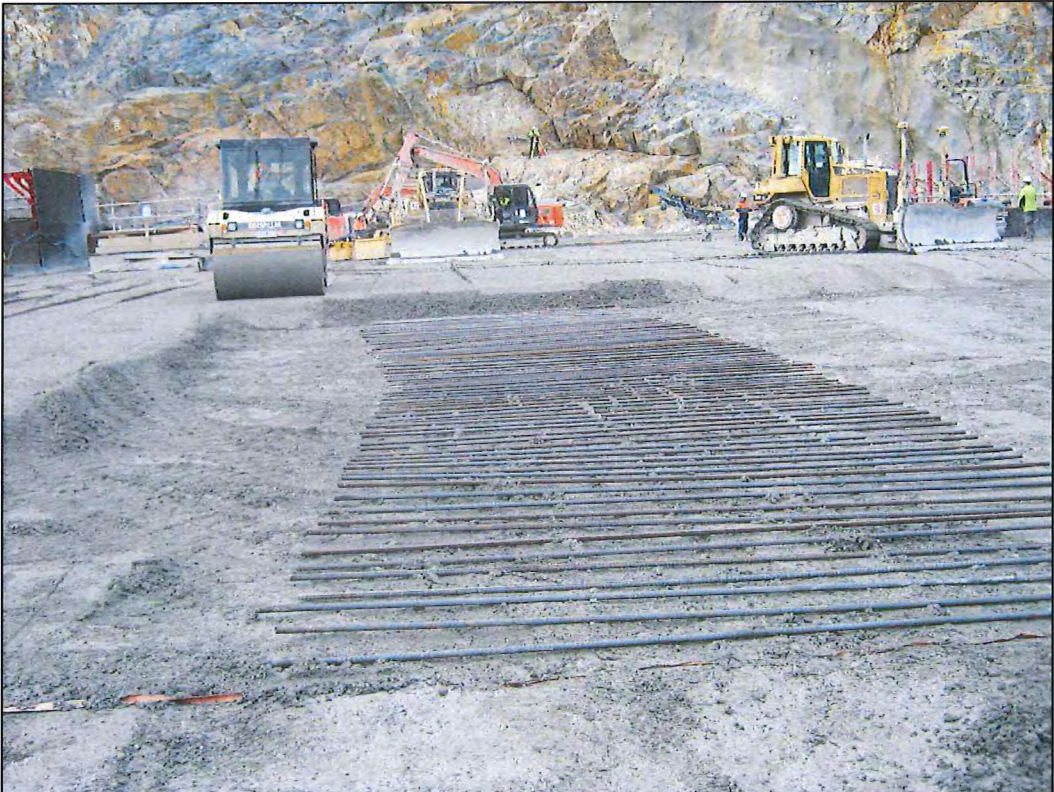
Photo D.7 – N28 reinforcement bars being installed on top of the cross valley cracks in Monolith G.
