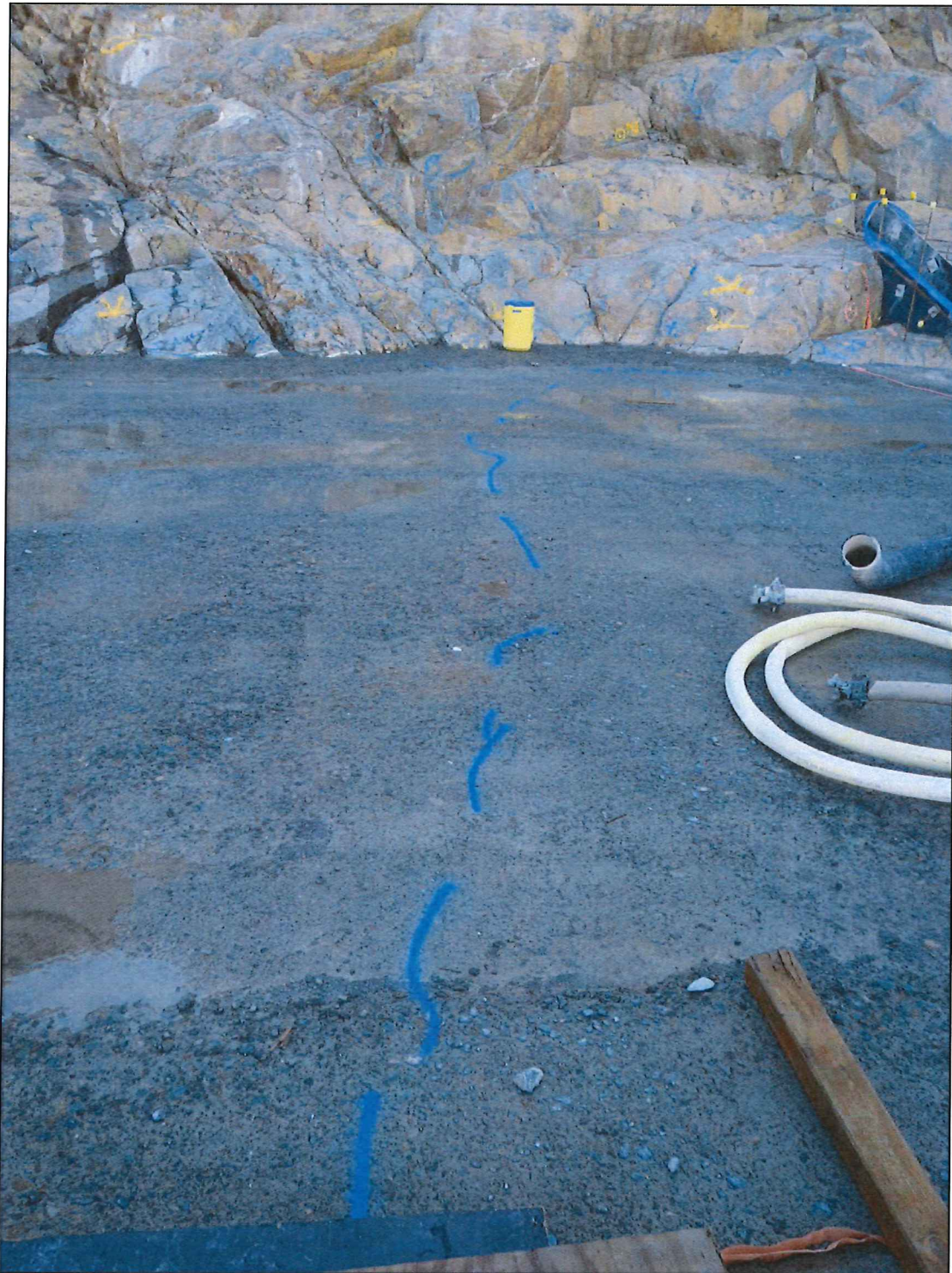
Photo A.1 - Cross valley crack in Monolith D. Taken looking towards left abutment.
