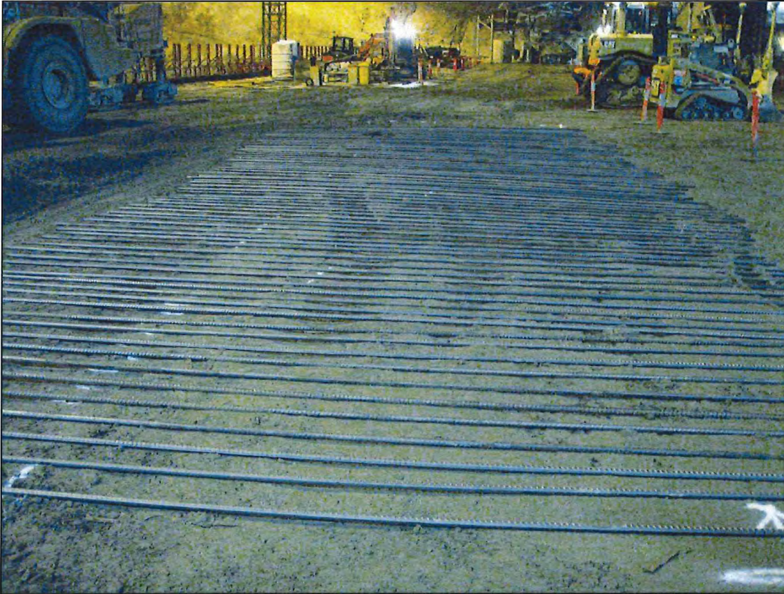
Photo D.10 N28 reinforcement placed abutment to abutment on cross valley cracks, shown here in Monolith G.
