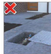
In driveway (unapproved)
