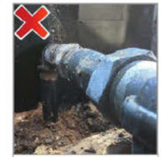
No copper risers
