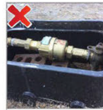
Incorrect meter height
