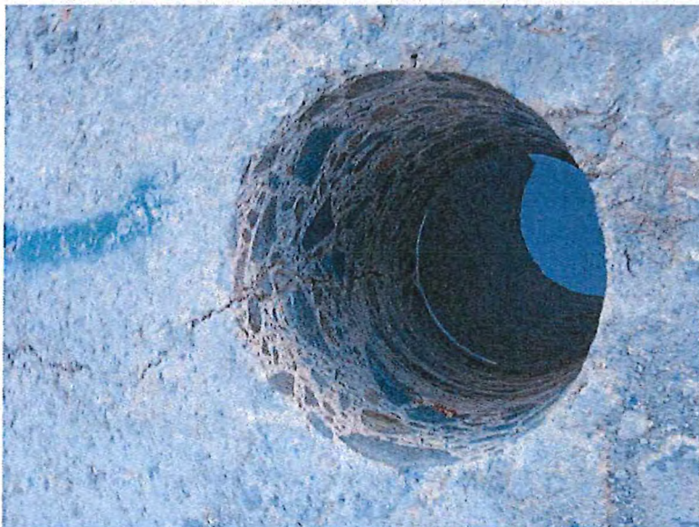
Photo 3 – 150mm core through upstream-downstream crack.
