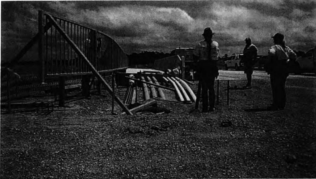
Image 03: Level issues with the transition of footpath and pedestrian handrail at bridge (RFI097A)
