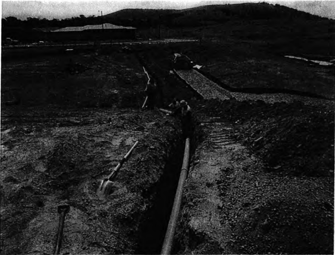
Installation of conduits for street light power supply from Casey sub station
