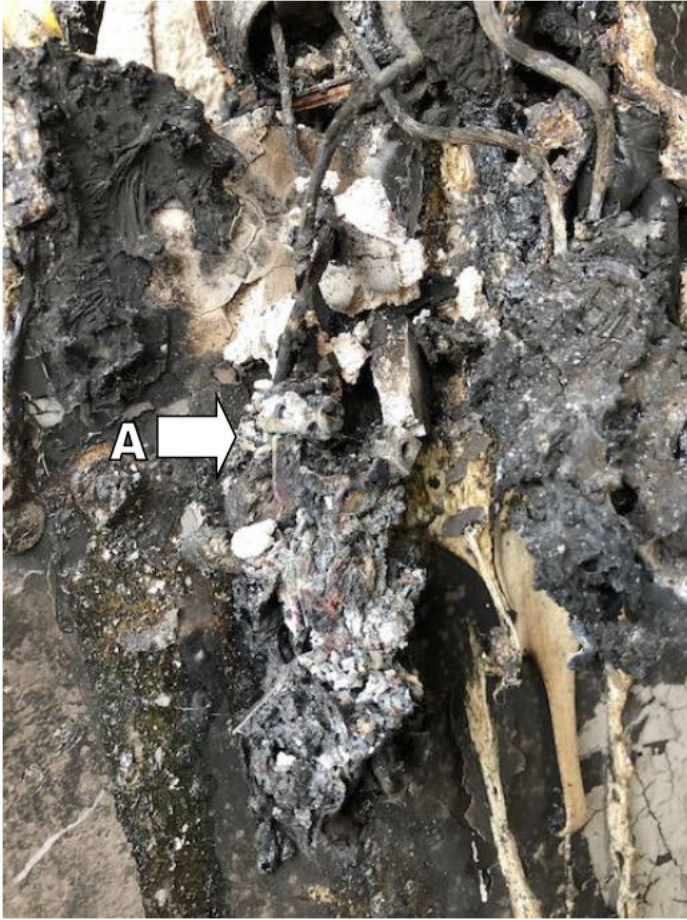
Closer view of Solar Array DC Isolator showing: A – Remains of DC cables with Isolator terminal attached
