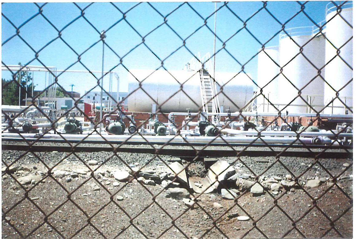
Photo 2: Unloading Point Showing Drain
