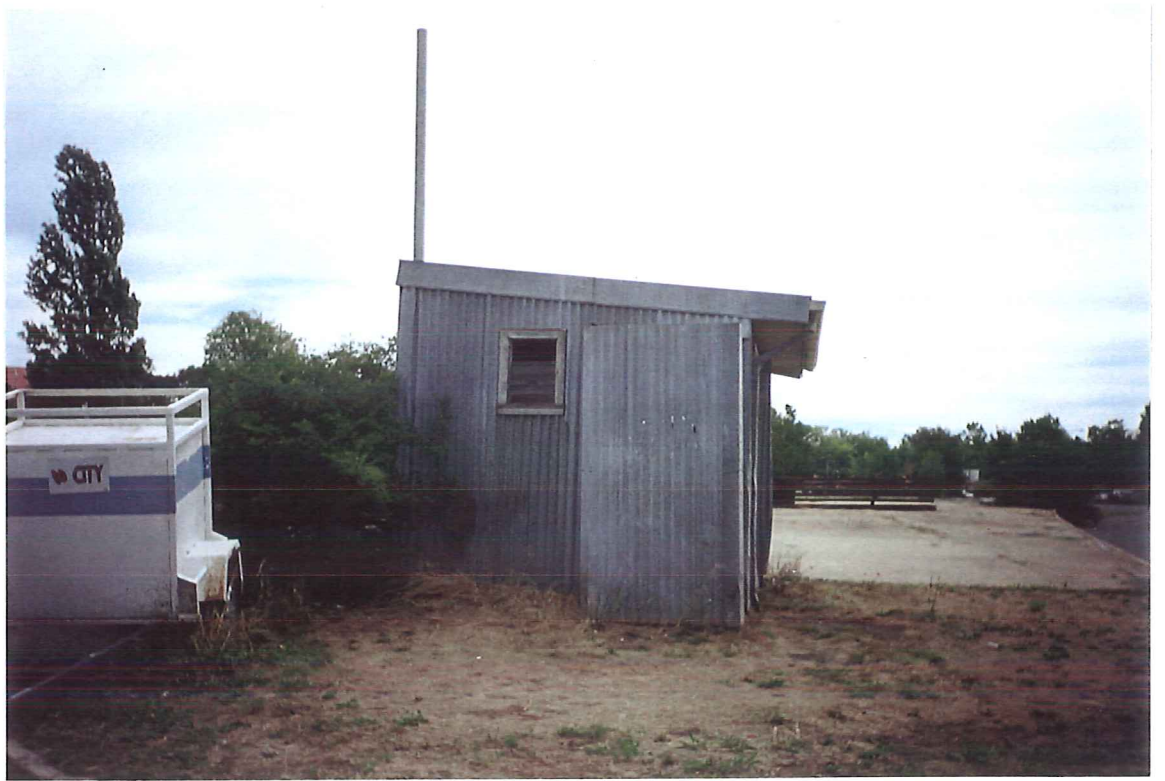
Photo 17: Toilet Shed with Asbestos Cement Debris Inside
