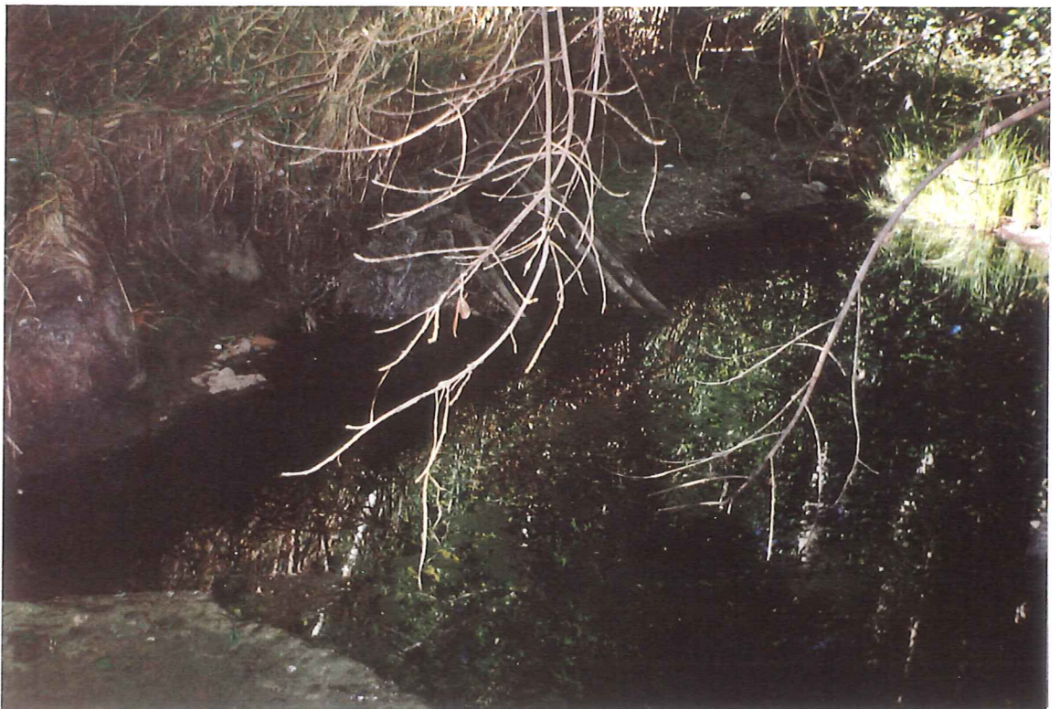
Photo 16: Oil Spillage in Stormwater Drain
