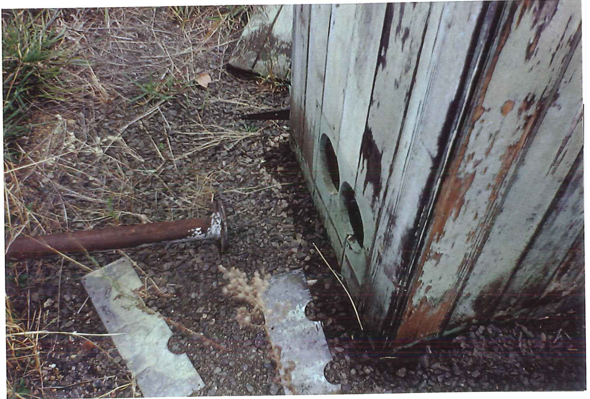
Photo 7: Staining Around Fuel Pump Shed
