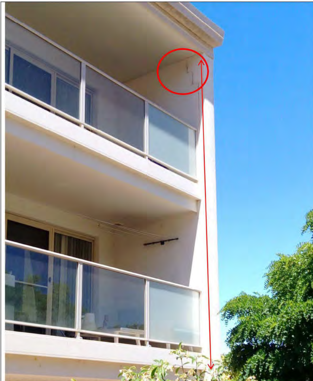
11. Render repair and vertical articulation joint required
