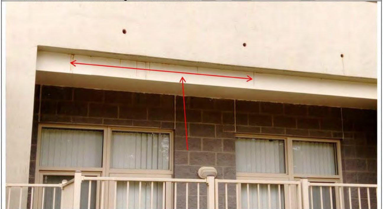
3. Minor corrosion showing on beam to unit 25
