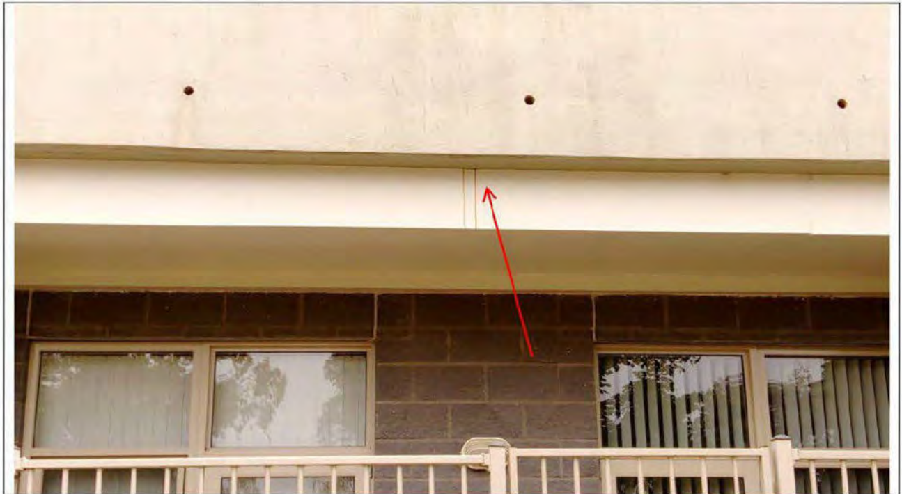
4. Minor corrosion showing on beam to unit 30
