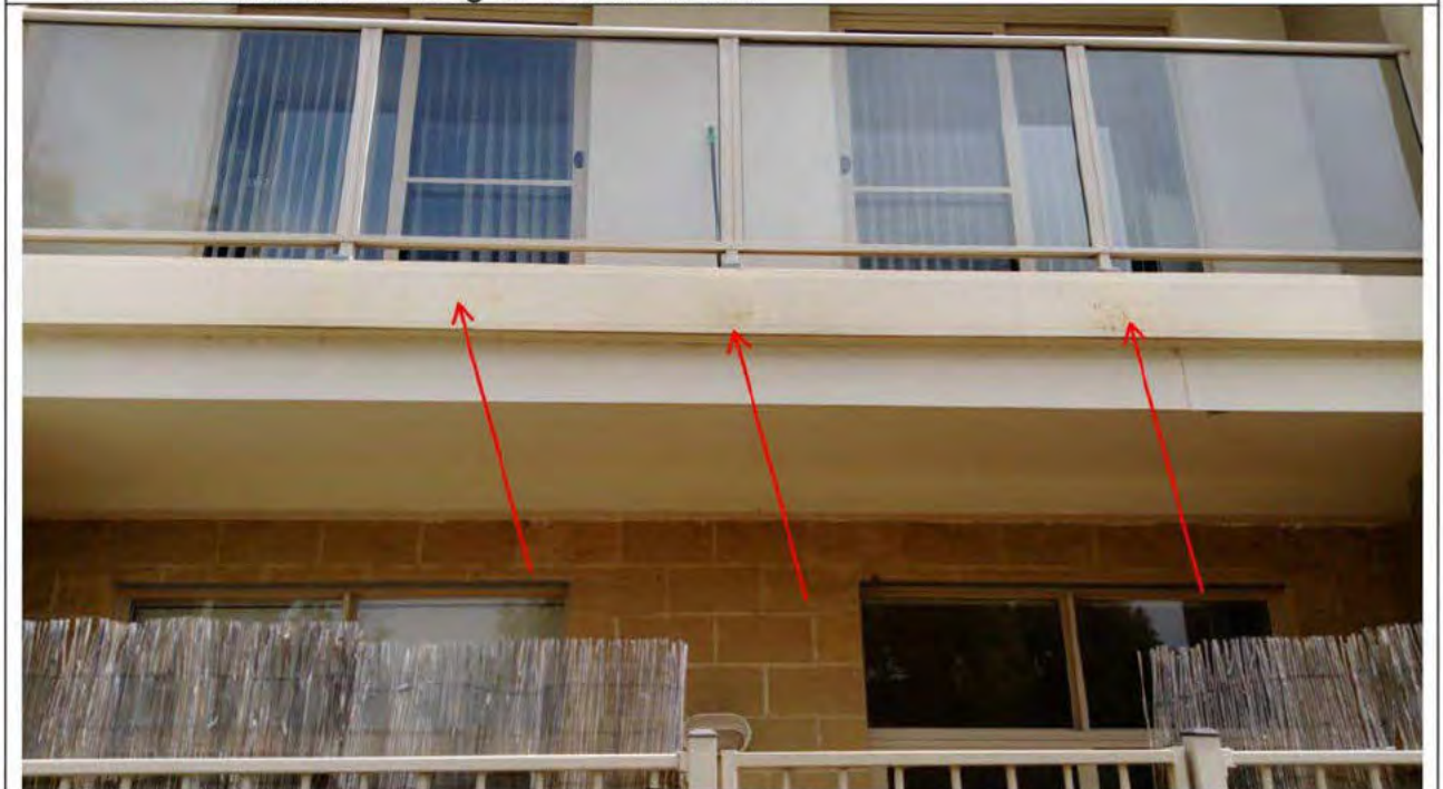
5. Minor face corrosion to unit 55 – considered to be a maintenance issue
