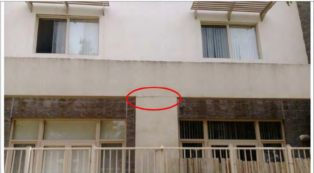
3- Typical minor articulation joint issue
