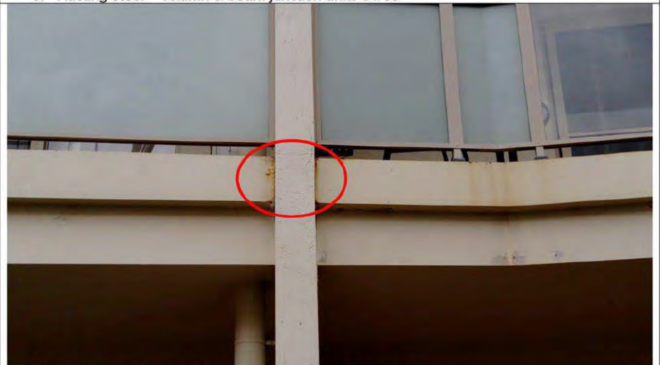
7. Rusting steel unit 42/48
