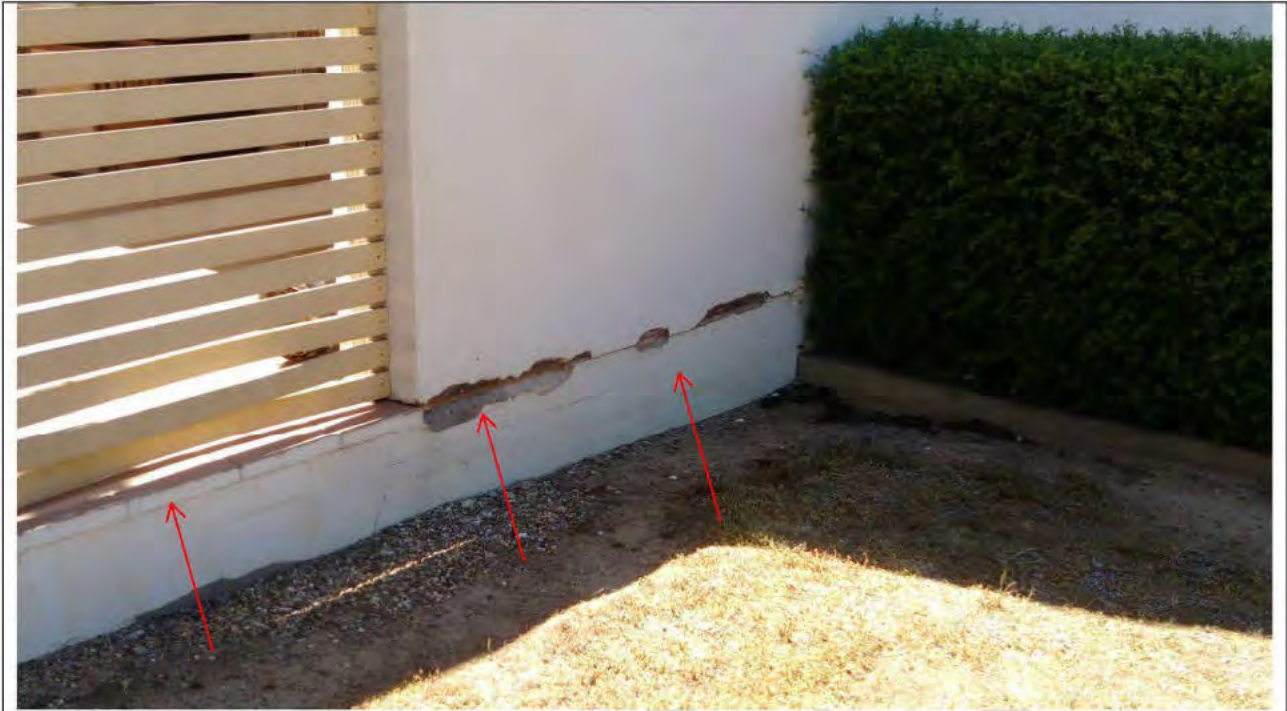
12. Buildin B - Horizontal slab edge render and articulation joints to be re-done
