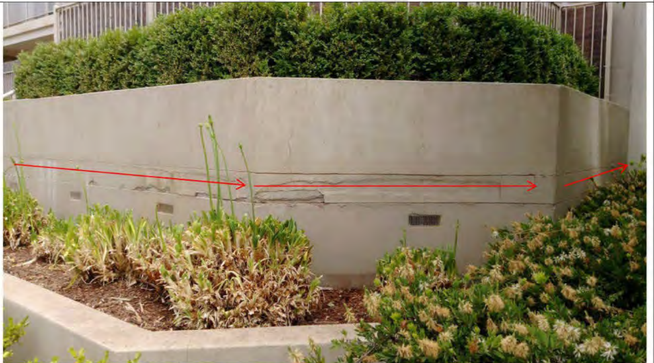
2- Failure at planter box Thynne st north end (block A). Render to be removed & replaced with adequate jointing between horizontal surfaces at the slab edges
