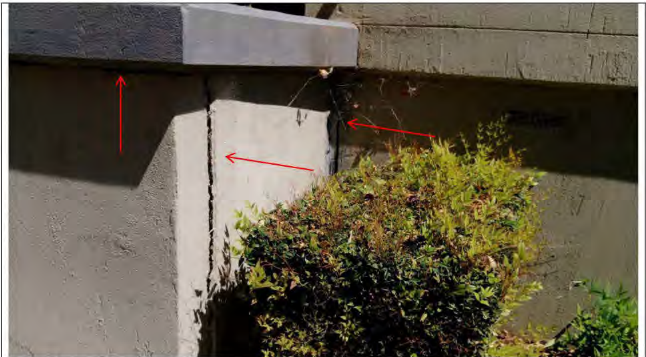
16. South block D – render repairs & jointing required
