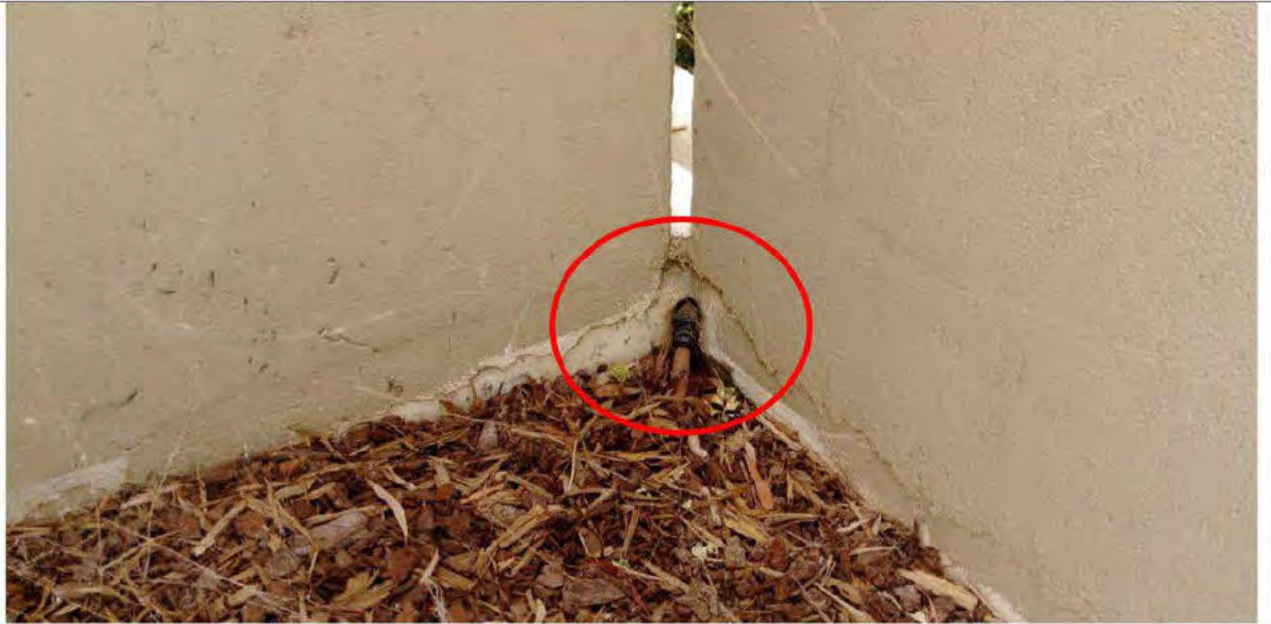
Irrigation penetration through planter to be sealed/waterproofed properly
