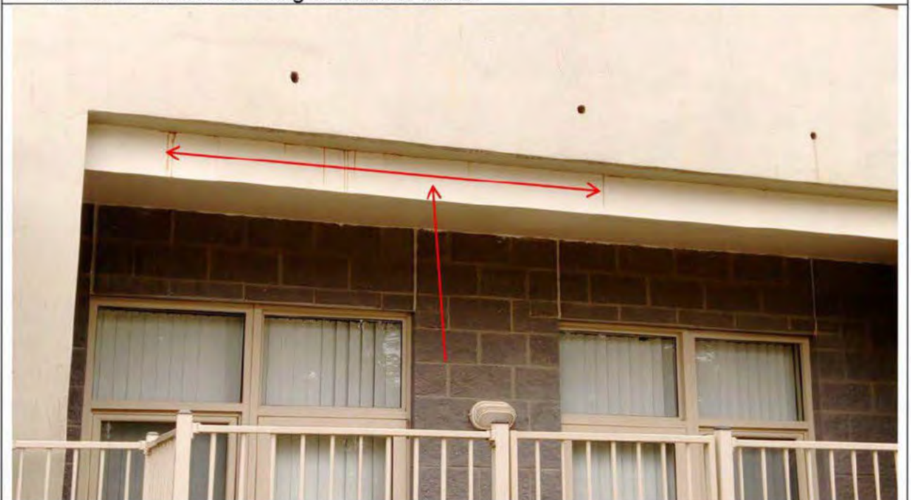
3. Minor corrosion showing on beam to unit 25
