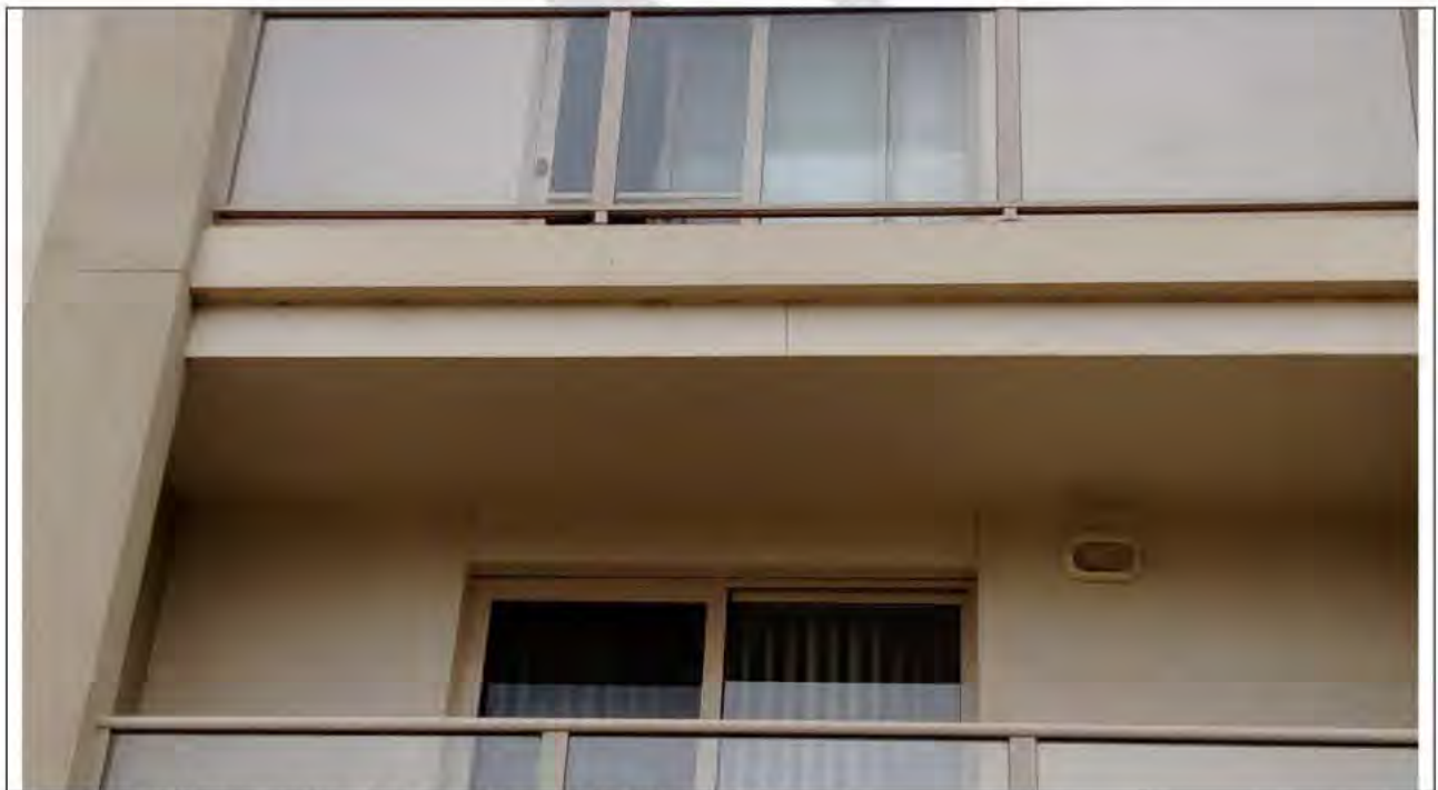
1. Slight corrosion (not visible on photo) unit 19
