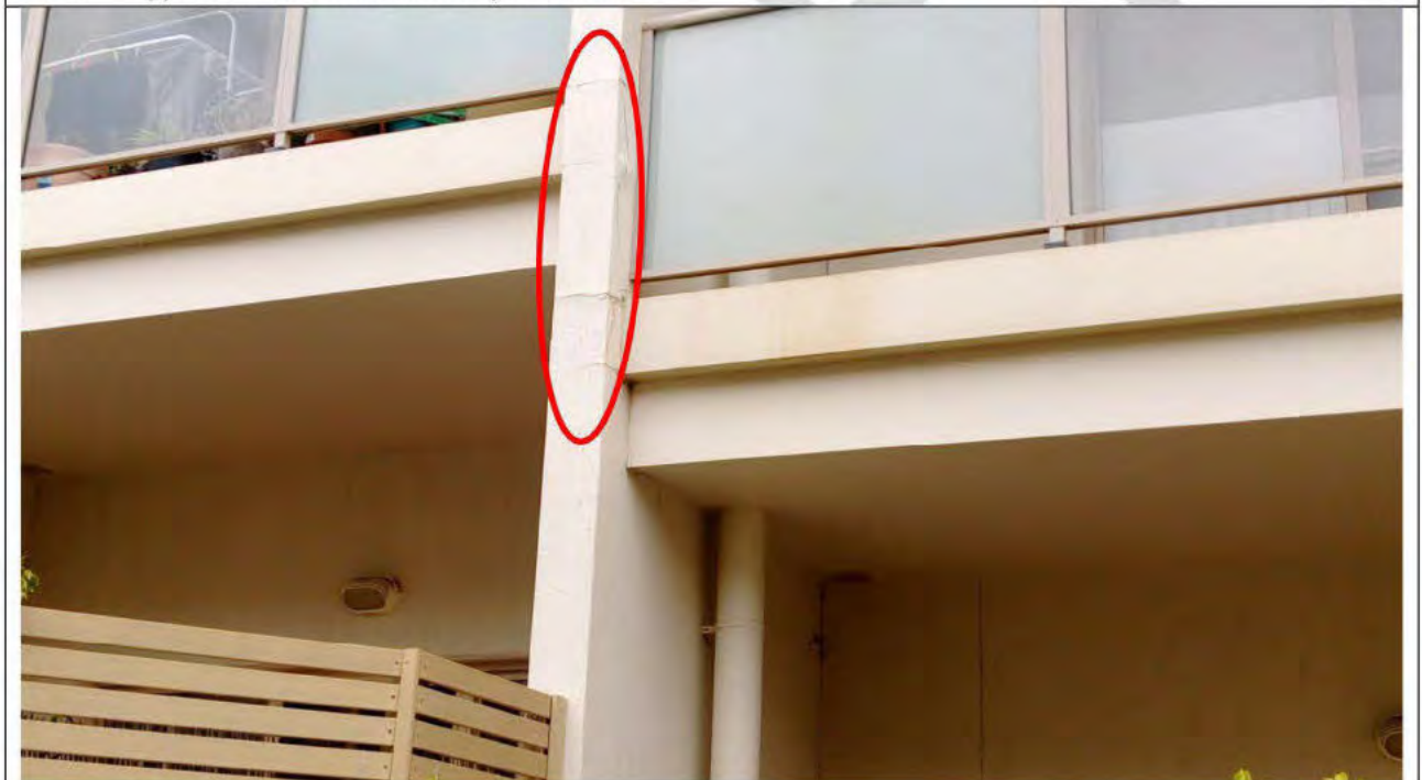
4- Render failure – unit 11/18
