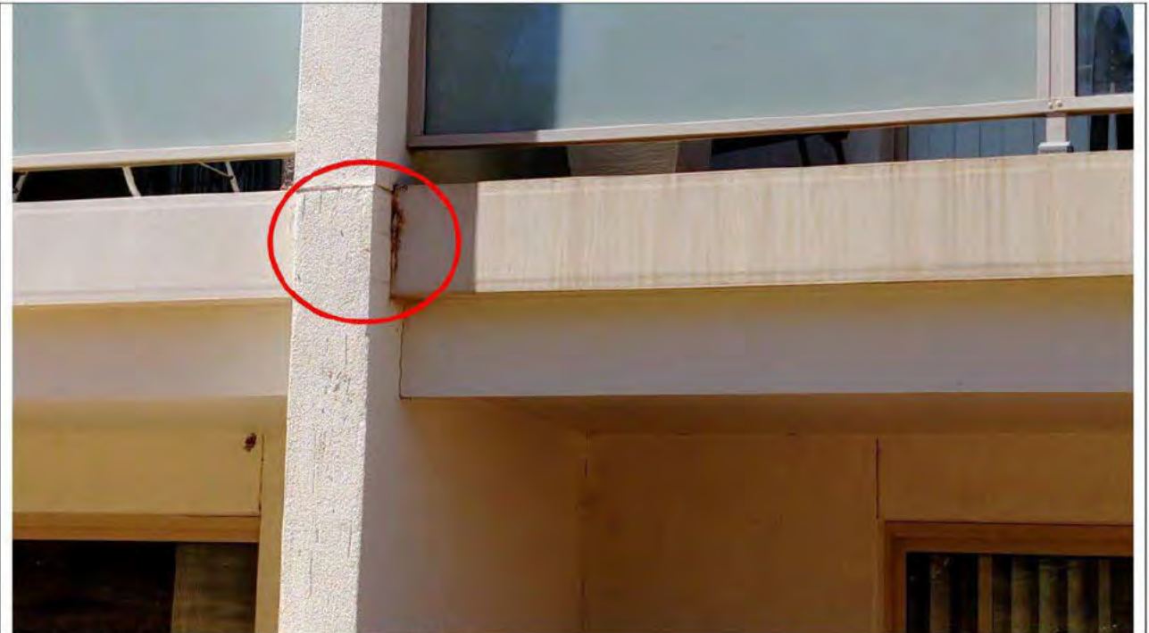
8. Minor beam corrosion – unit 75
