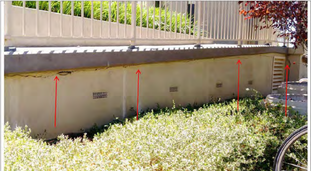
10. Horizontal render cracking to be cut out, repaired & flexibly sealed between top of wall & underside of slab Building B
