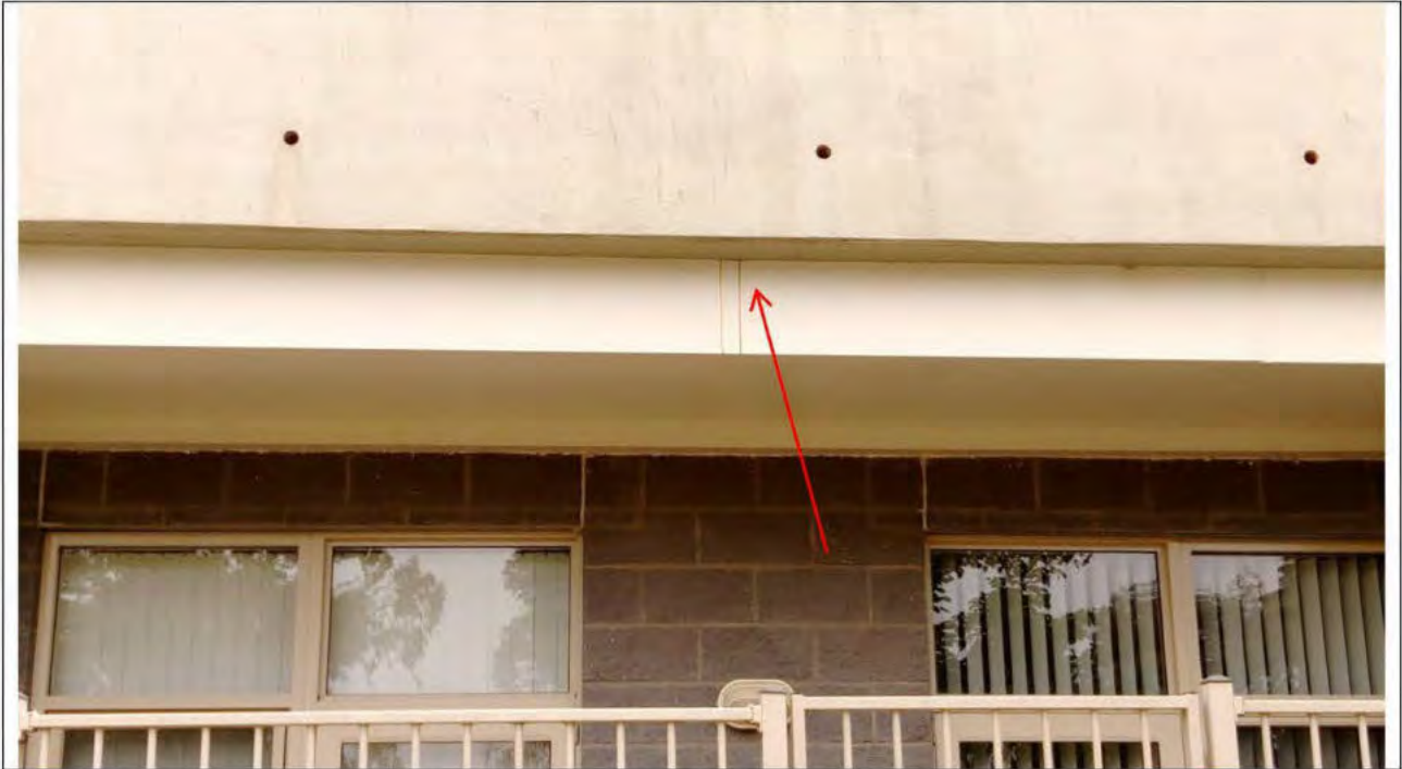
4. Minor corrosion showing on beam to unit 30
