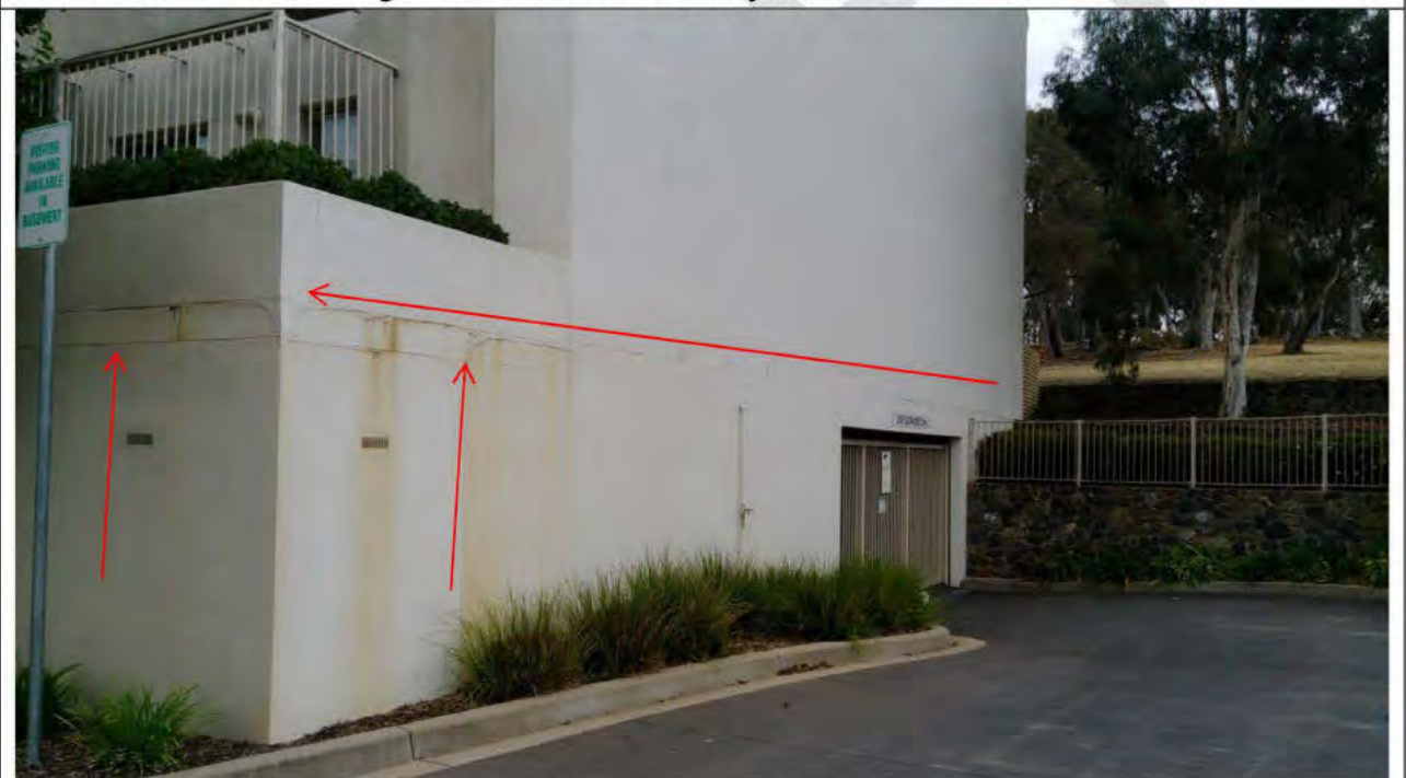
9. Horizontal slab edge render and articulation joints to be re-done
