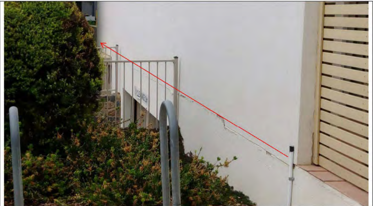
8. Horizontal slab edge render and articulation joints to be re-done
