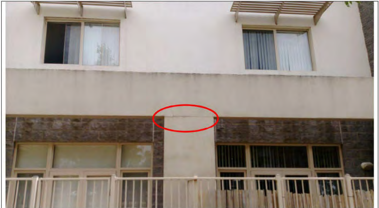
3- Typical minor articulation joint issue
