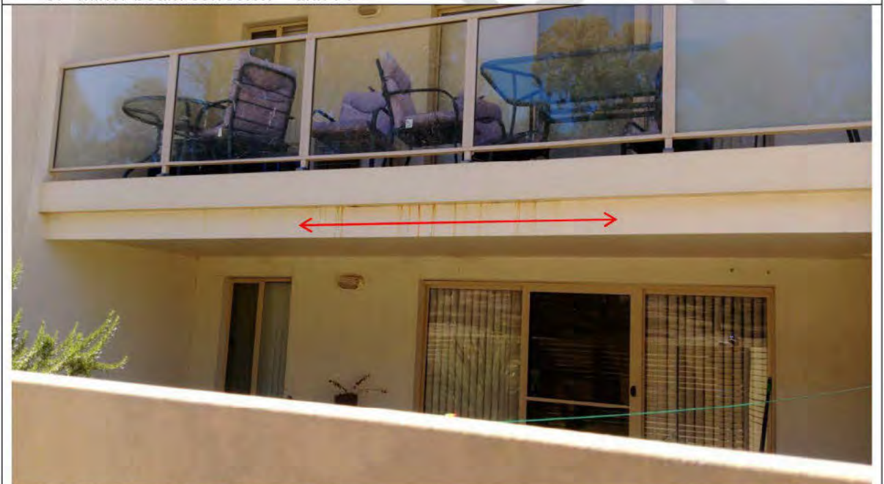
9. Minor beam corrosion unit 105
