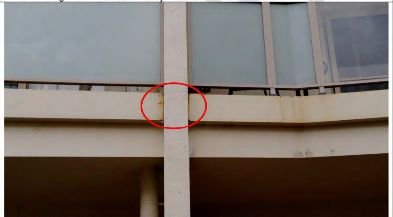
7. Rusting steel unit 42/48
