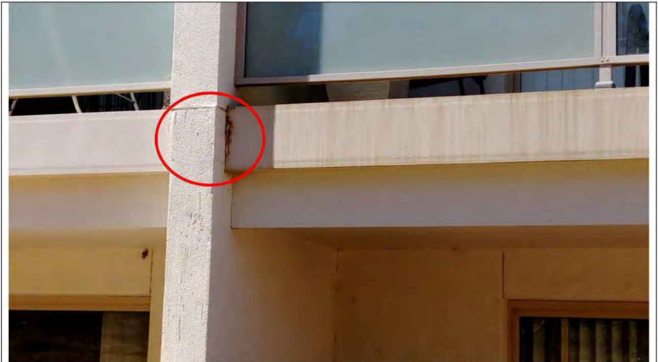
8. Minor beam corrosion – unit 75
