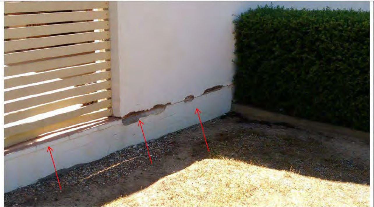
12. Buildin B - Horizontal slab edge render and articulation joints to be re-done
