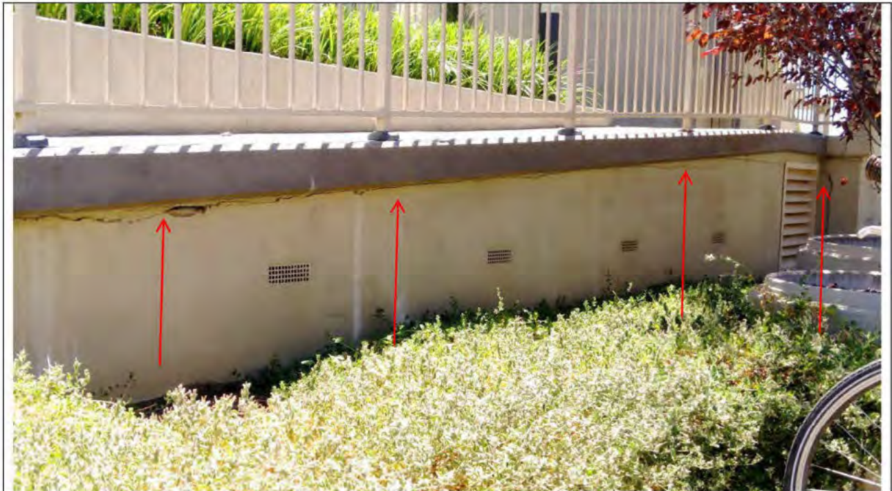
10. Horizontal render cracking to be cut out, repaired & flexibly sealed between top of wall & underside of slab Building B
