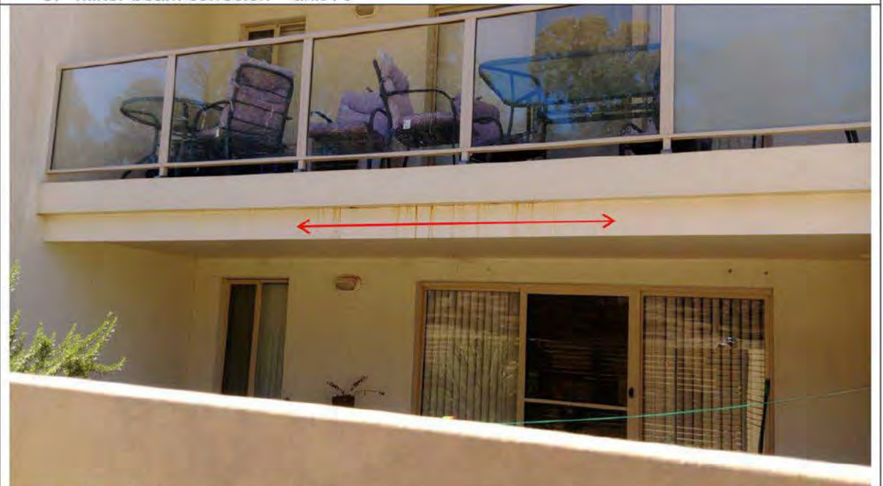
9. Minor beam corrosion unit 105
