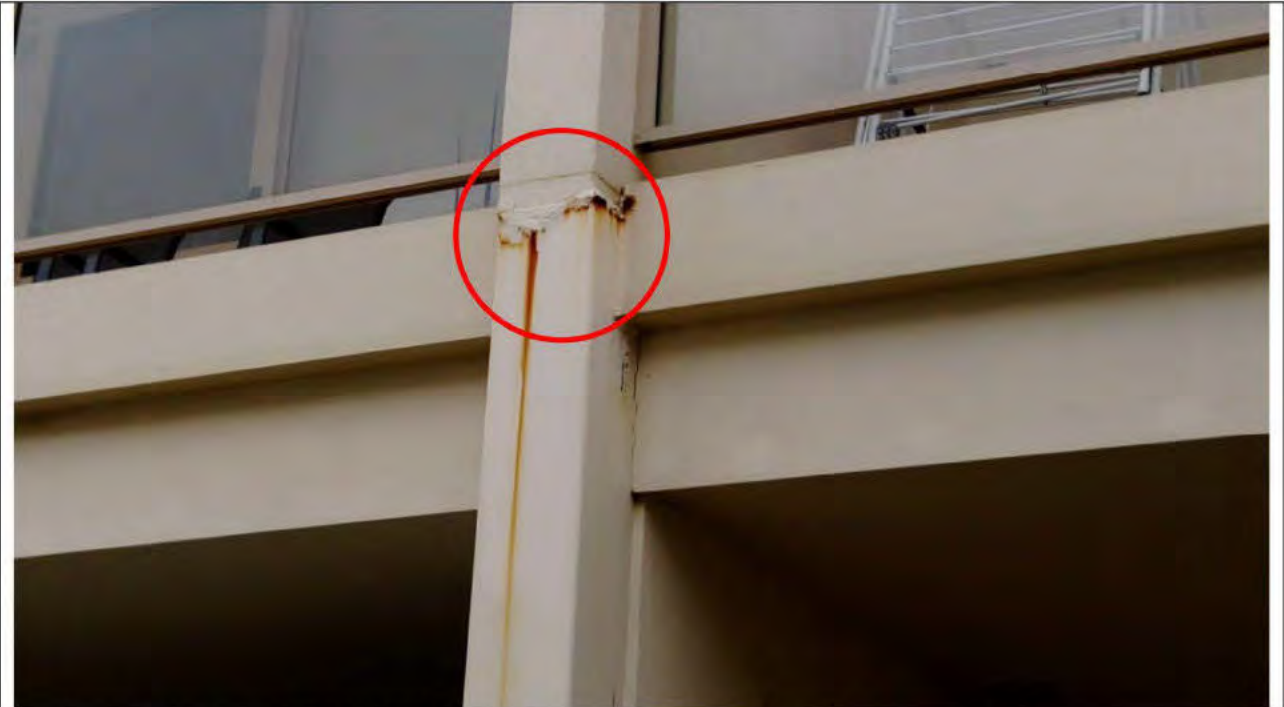
6. Rusting steel – column & beam junction units 31/36
