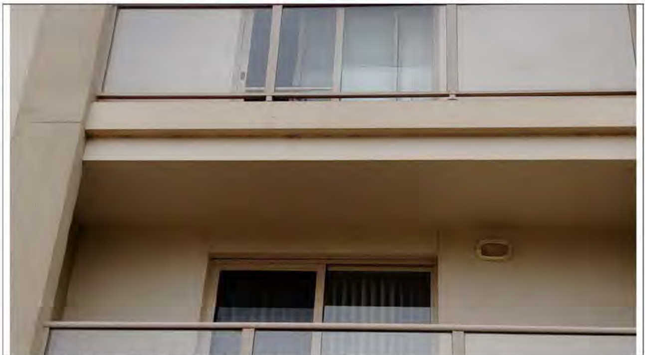
1. Slight corrosion (not visible on photo) unit 19
