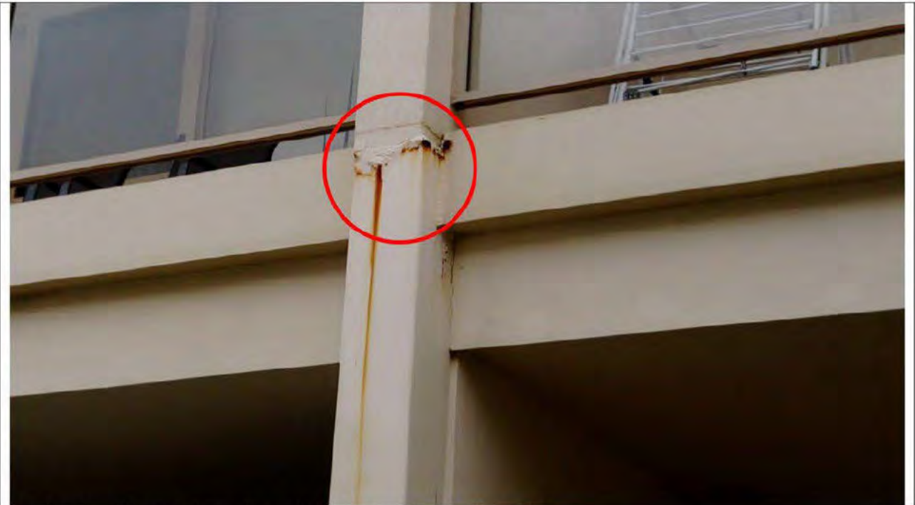
6. Rusting steel – column & beam junction units 31/36
