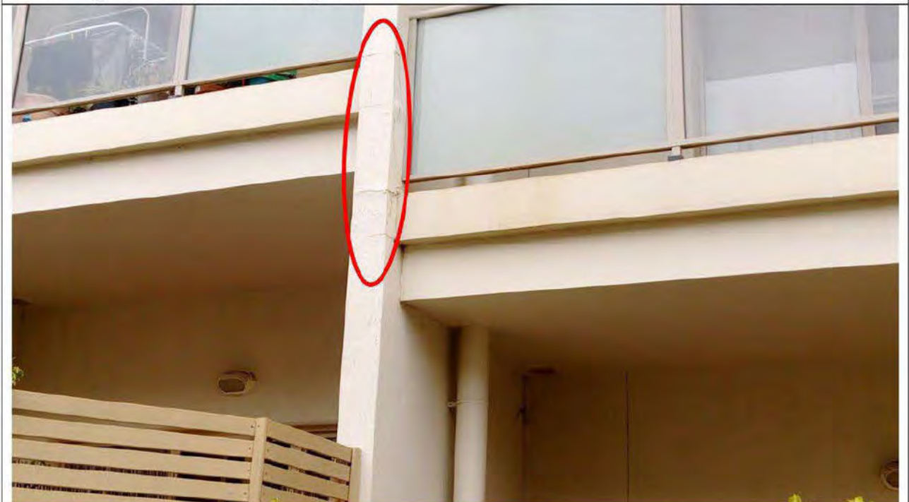
4- Render failure – unit 11/18
