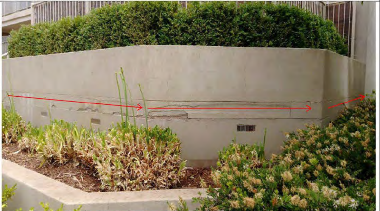
2- Failure at planter box Thynne st north end (block A). Render to be removed & replaced with adequate jointing between horizontal surfaces at the slab edges
