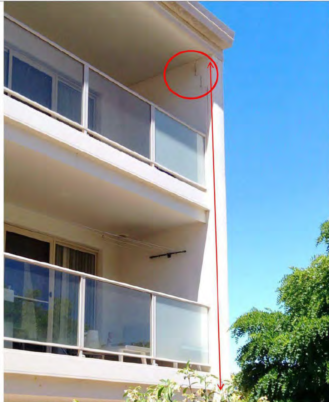
11. Render repair and vertical articulation joint required
