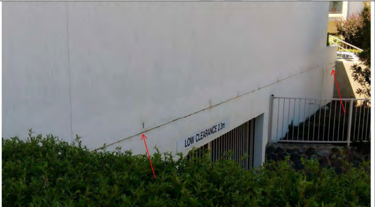
13. Building B - Horizontal slab edge render and articulation joints to be re-done – weepholes to be cleaned out
