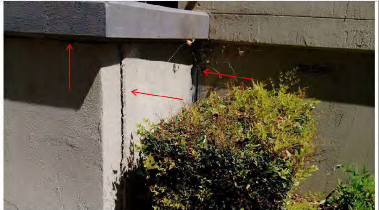
16. South block D – render repairs & jointing required
