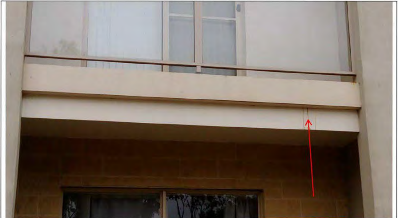
2. Minor corrosion showing on beam to unit 24
