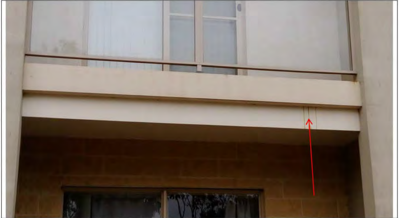
2. Minor corrosion showing on beam to unit 24
