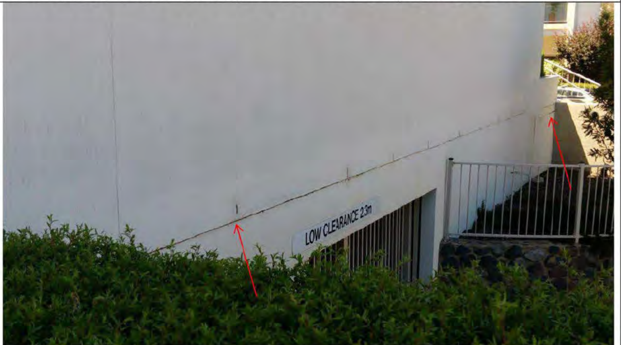
13. Building B - Horizontal slab edge render and articulation joints to be re-done – weepholes to be cleaned out
