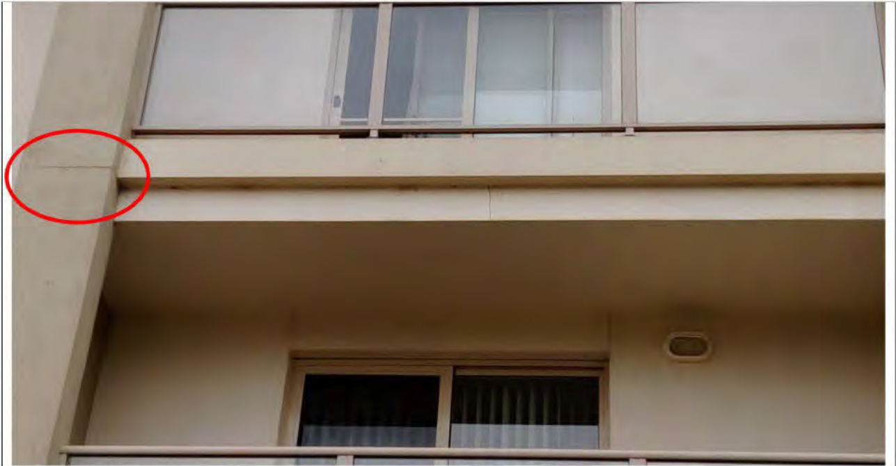
1- Typical minor articulation joint issue
