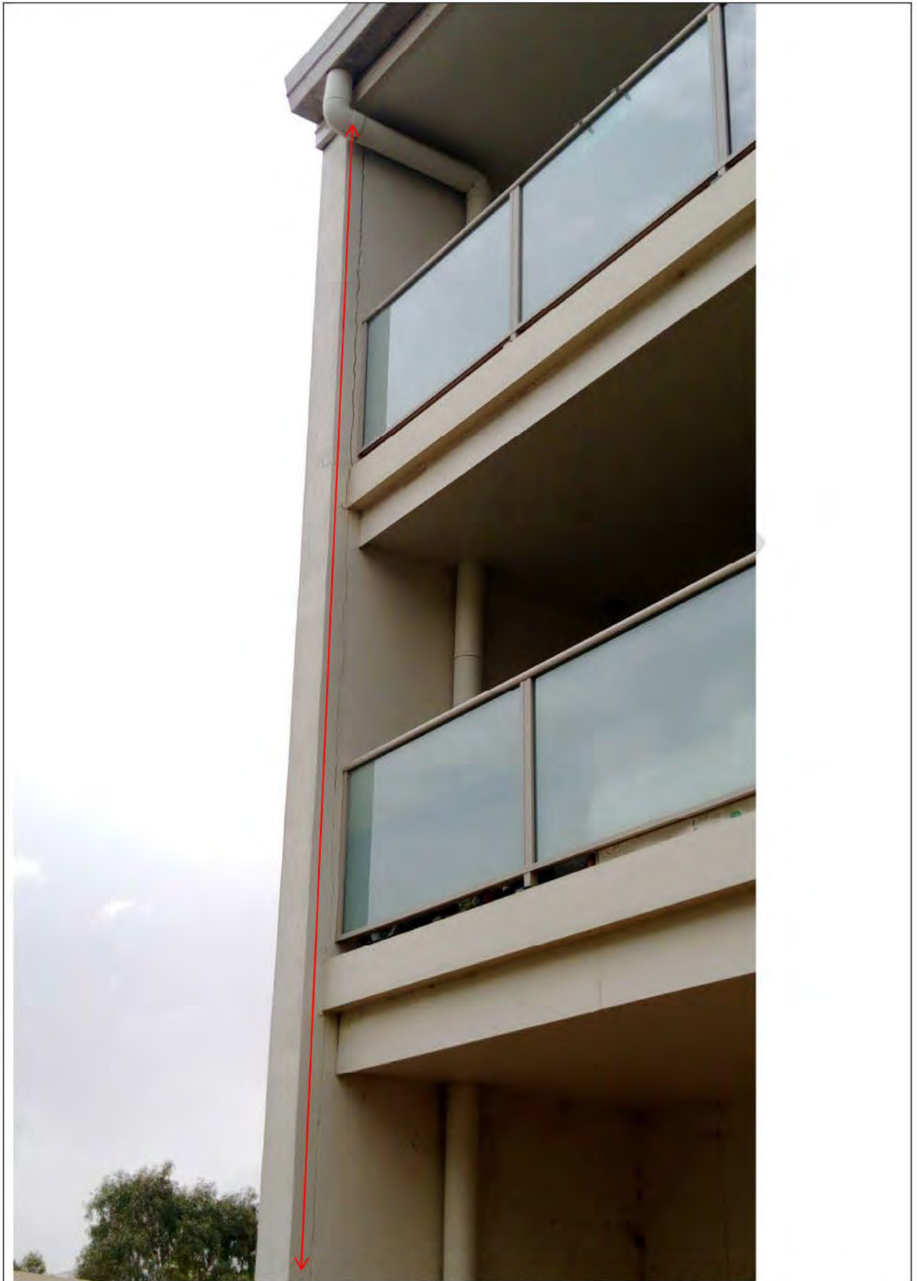
15. Block D East - Vertical articulation joint, repairs & sealant required
