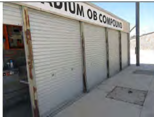
Corrosion to steel columns.
