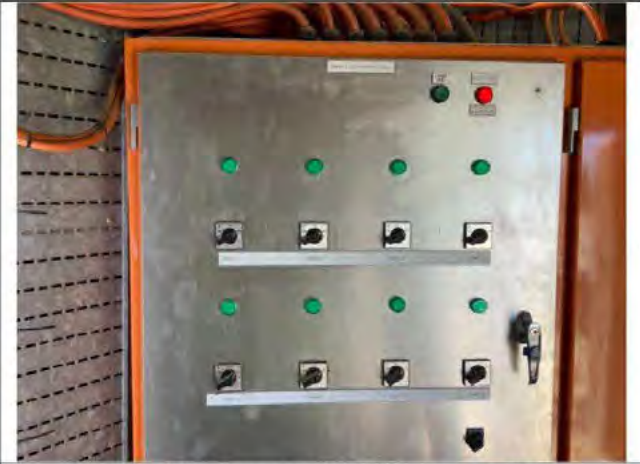
Typical light tower MSB Control section.
