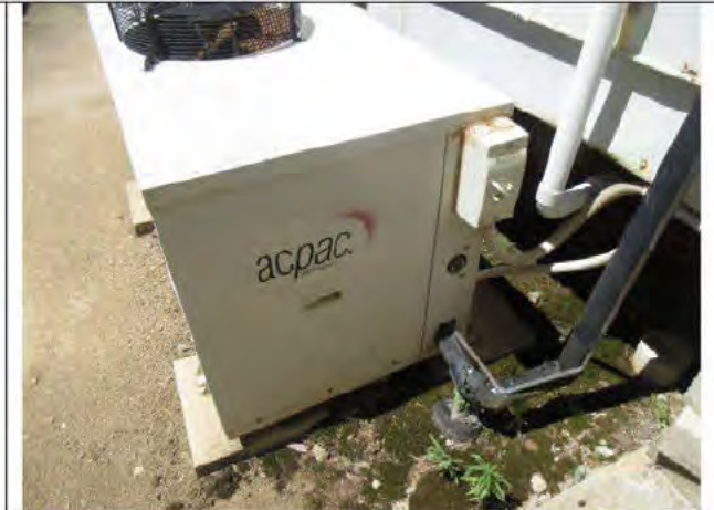
Typical external compressor/condenser serving Food Concessions.
