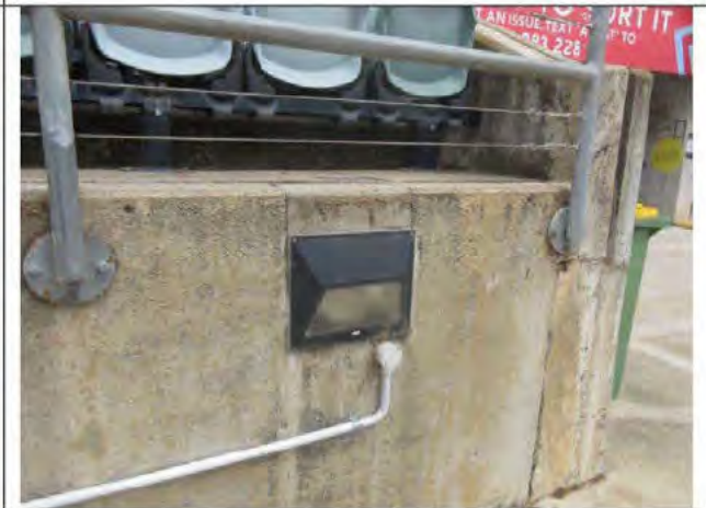
Typical luminaire to base of terraces.
