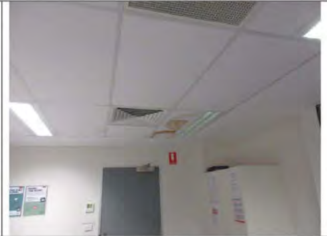
Moisture damaged ceiling tiles to West Ticketing Office.
