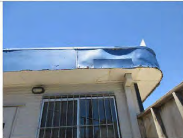
Damaged FC cladding to K9 Food Concession.
