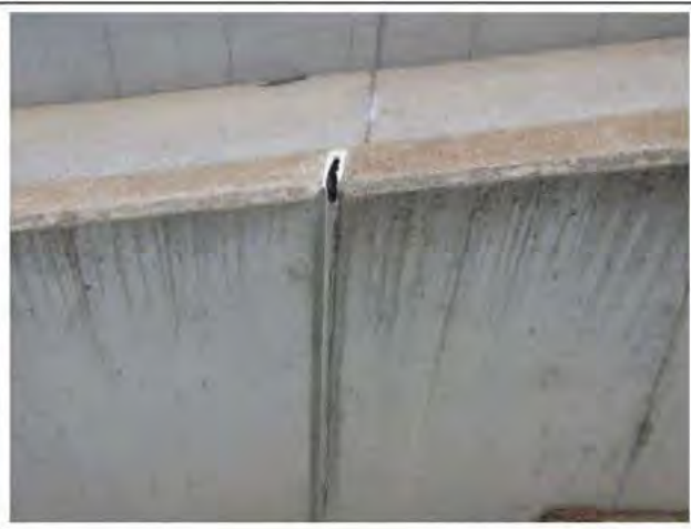
Deteriorating sealant to perimeter concrete wall expansion joint
