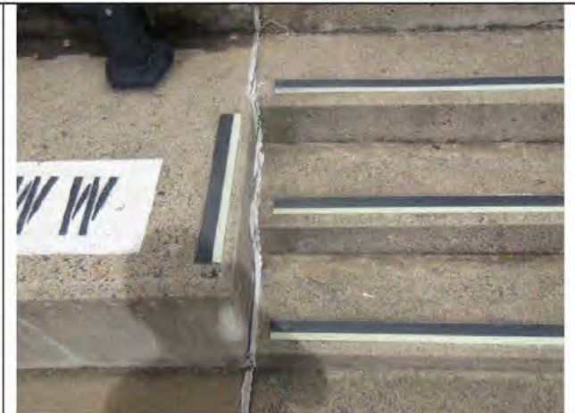
Degrading sealant expansion joints to the South Terrace.
