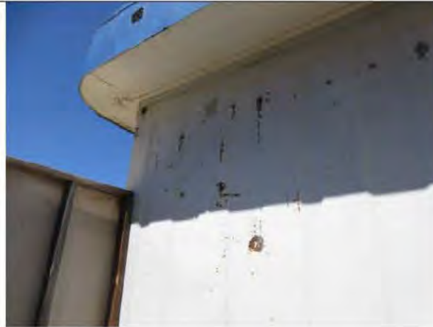
Degradation of coating and minor surface corrosion to container walls.
