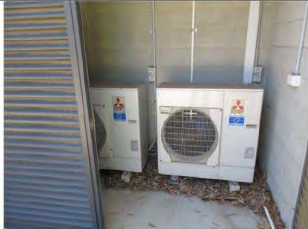
AC Condensers serving the West Ticketing Office.
