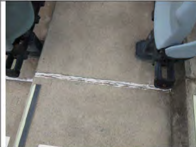
Typical example of deteriorated sealant expansion joints.
