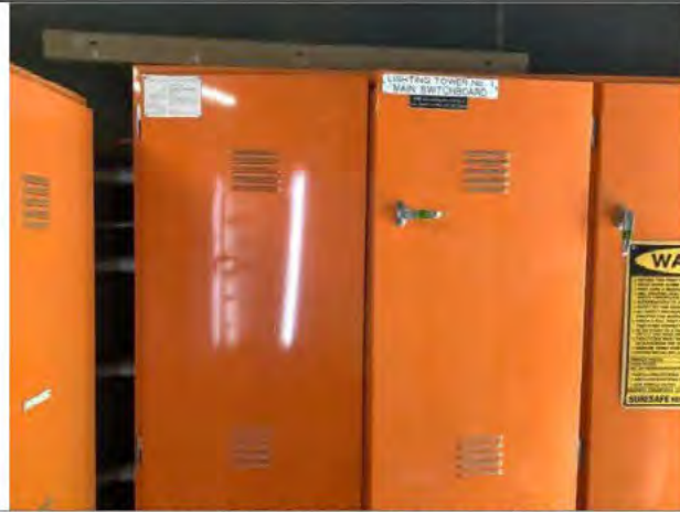
Typical view of switchboard serving light towers.
