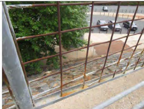
Rear balustrading/fencing to the top of the terraces corroded.
