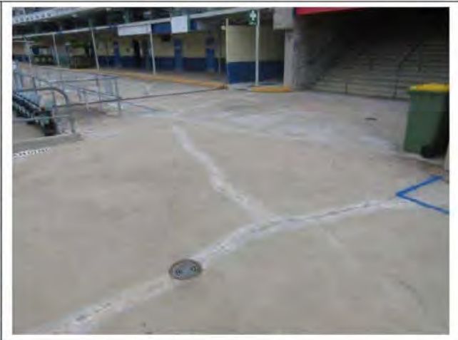
Cracking and evidential historic repairs to north-west corner of concourse.
