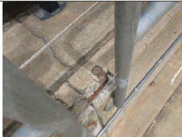
Damaged concrete and exposed steel reinforcing.
