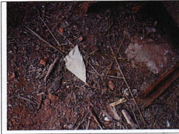
Photograph 17: Between tall chimney & K3 – Debris to ground & scattered throughout site Sheet Refer Sample: M0102
