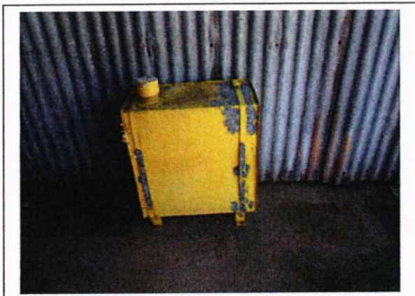
Photograph 35: Portable AST to building M3
