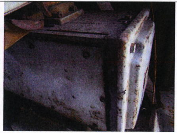
Photograph 22: M3 - Mastic to original distribution board Refer Samples: 3617 – 103 – A6
