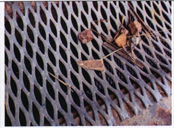
Photograph 18: Front of B - Moulded sheet debris to ground & throughout site Refer Sample: M0103
