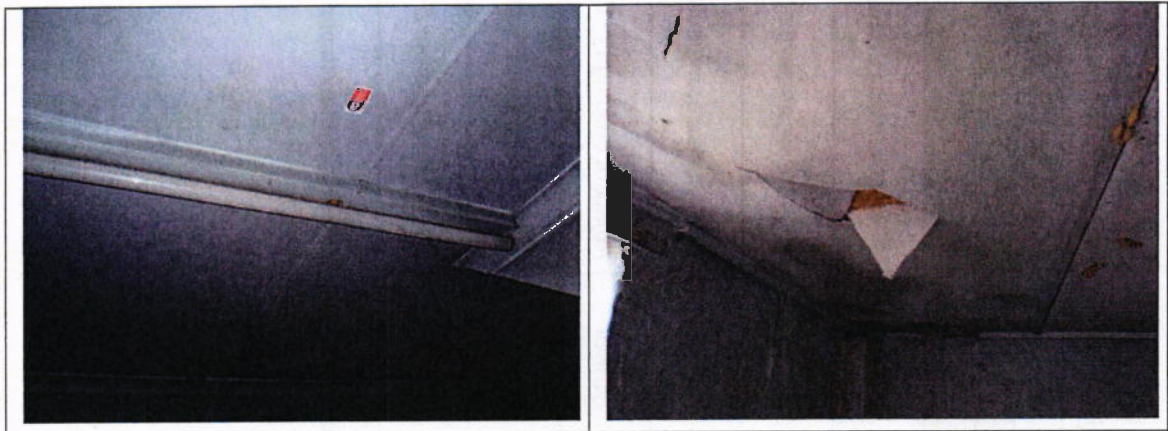
Photograph 3: Former canteen - Ceiling sheet Refer Sample: 2810 – 40 – A5
