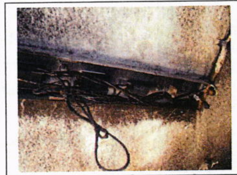
Photograph 31: Building SS2 Metal – Unidentifiable due to fire damage
