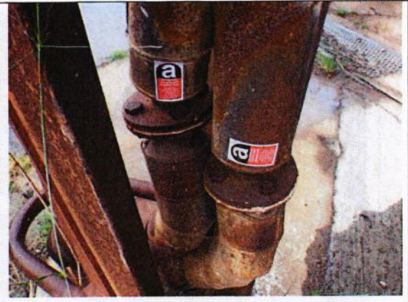
Photograph 10: B - Front corner, gaskets adjacent downpipe Refer Sample: 3617 - 103 - A4
