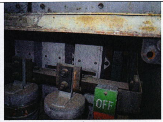
Photograph 12: M2 & M3 - Flash guards to distribution board Refer Sample: 3617 - 103 - VA1
