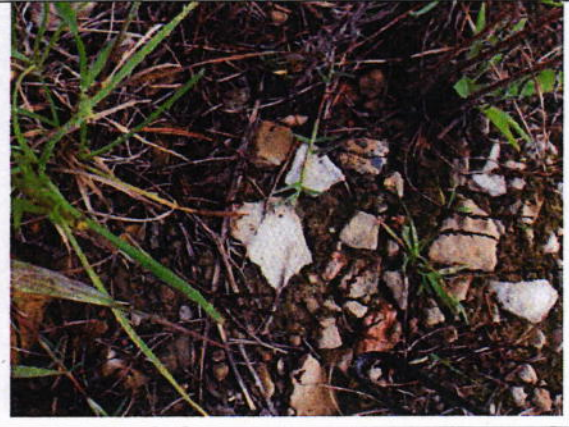
Photograph 14: Adjacent bridge to K2 - Debris to ground Refer Sample: M0099 (b)
