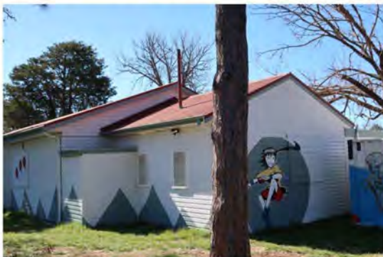
Figure 38: South-west corner, with 1955 skillion section (centre) and gable addition (1955 and 1985) in foreground
