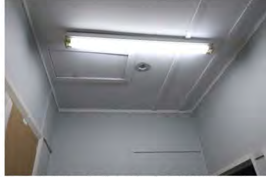
Figure 41: Battered ceiling and walls to 1955/1985 section
