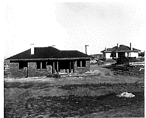
Figure 2.6 Cottages under construction in Oakley and Parkes, c.1925 Source: National Archives of Australia
