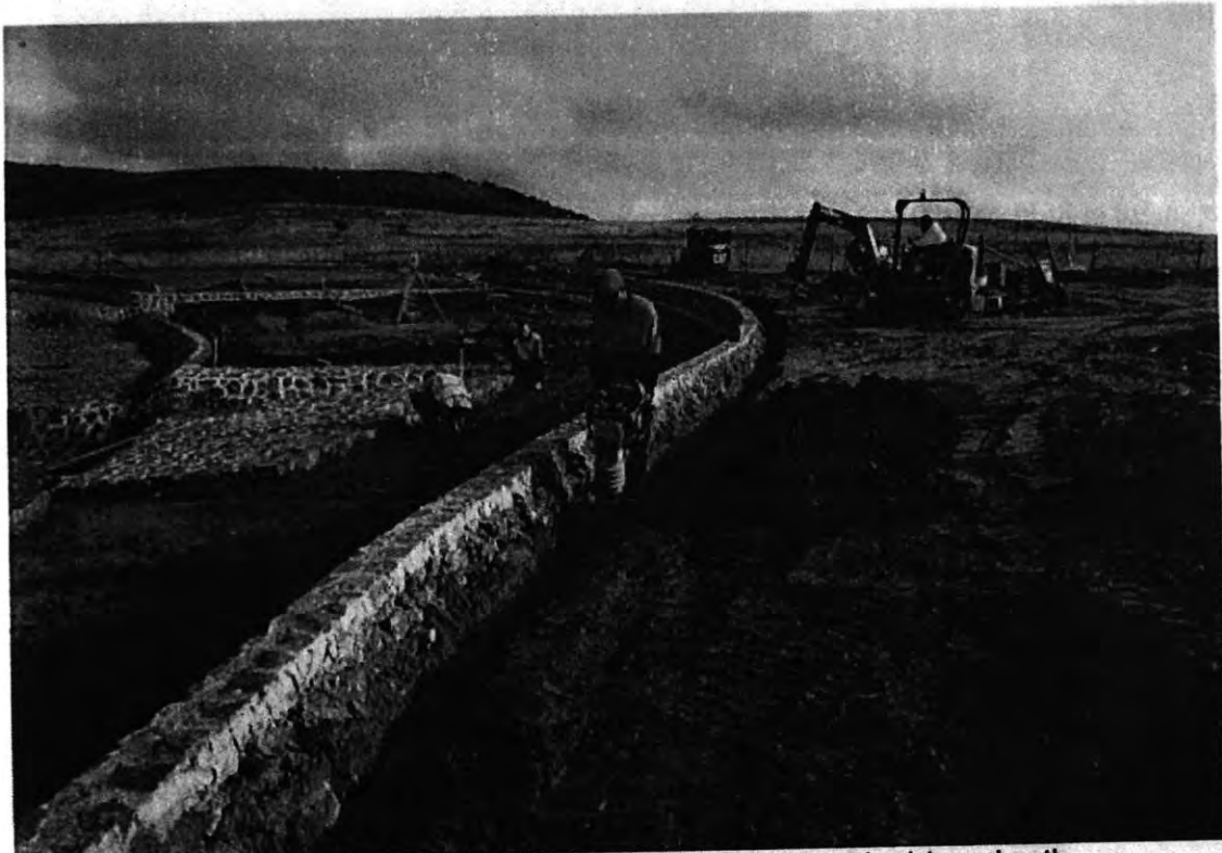
Back filling against the stone pitched retaining wall at the equestrian/shared path
