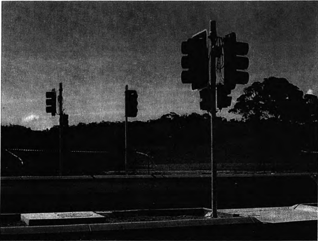
Traffic lights at Mirrabai Drive
