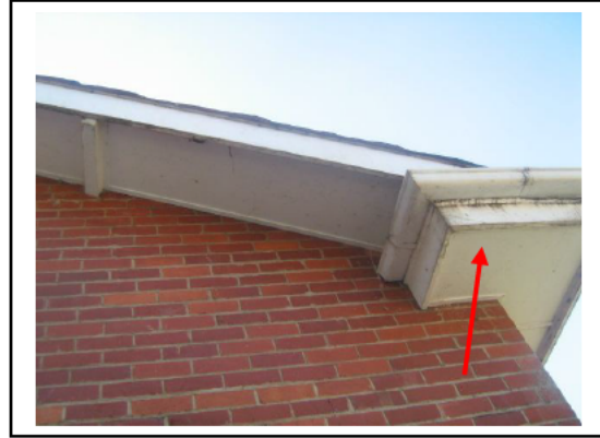
Photograph 2: Southeast corner of building – eave sheet (refer sample no. 3971 – A8).
