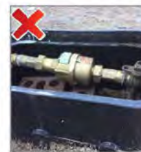
Incorrect meter height
