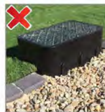
Incorrect box level
