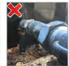
No copper risers
